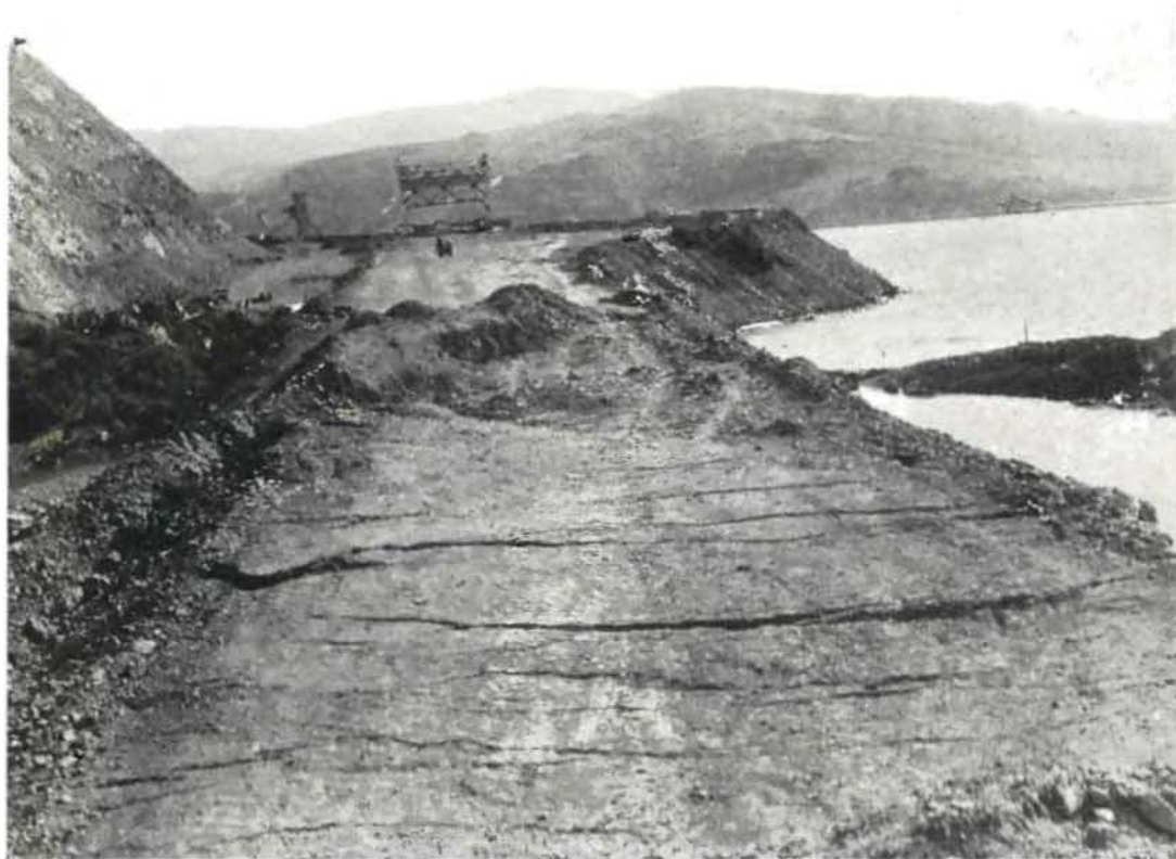
SLOUGH OF DESPOND , this was for the engineers until they got mad and dynamited the fill that wouldn't fill on the newly-opened Alto-Waldo link of the Redwood Empire highway across an arm of Richardson Bay. Note the cracks showing the settling despite repeated dumping of hundreds of tons of road material. Tons of explosive finally blasted the way to hard bottom.
