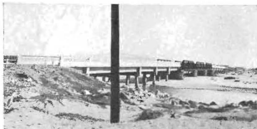
PONY TRUSS spans of steel carried coast traffic over the old inadequate 24-foot bridge across the Santa Ana River in Orange County.
