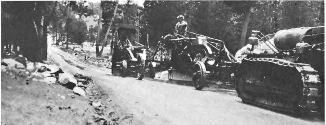
MODERN OUTFITS of the Division of Highways composed of tractor and grader team up in the preparatory work of leveling the road for the oil treatment and covering and mixing the oiled surface material.
