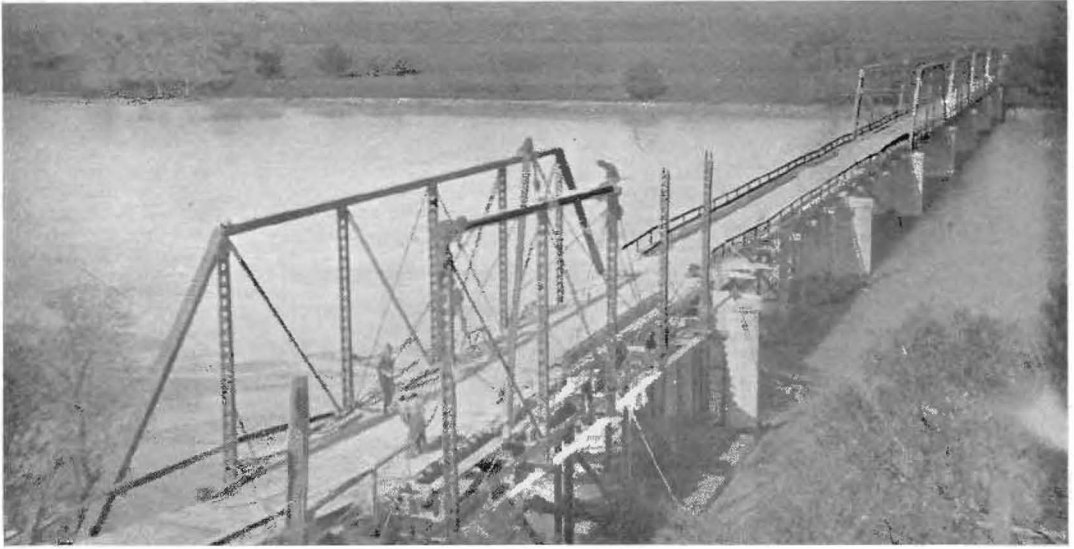
DECREPIT AND DANGEROUS , this old bridge on the Coast Route over the Salinas River at Bradley, with its 15-foot roadway, shaky wooden spans and sharply curved end, has been supplanted by a modern structure.
