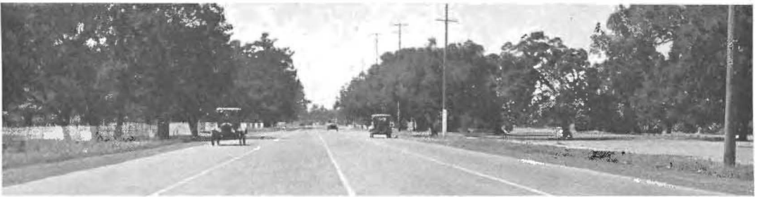
NO WRINKLES or rough places are to be found in this fine forty-foot asphalt concrete pavement laid in Santa Clara County under superior mix formulas and finishing methods developed in the Public Works laboratory.
