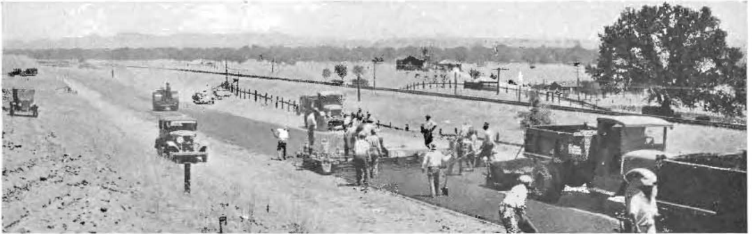
LIKE A CARPET this big gang laid a broad strip of asphalt concrete pavement in San Luis Obispo County in record time by employing more efficient methods developed by State experts.
