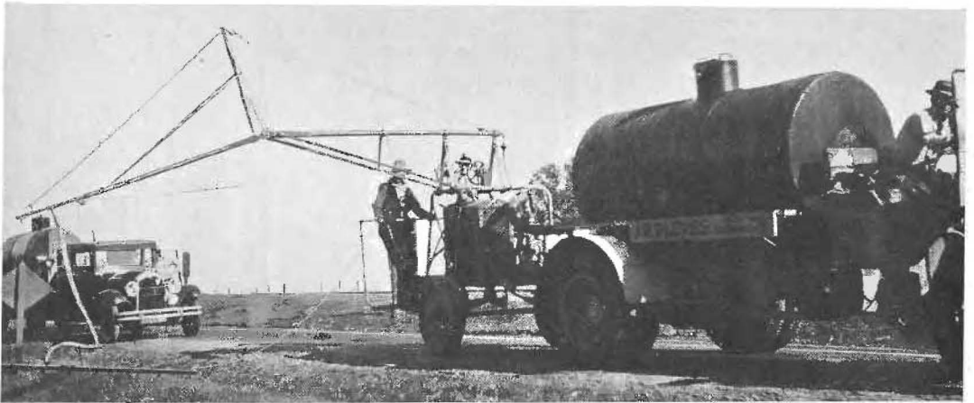
THE TANK CORPS with numerous units equipped like the above is engaged in the annual preliminary skirmish against old Demon Fire Hazard on all State highways. A weed spraying outrigger on an oil spreading trailer makes combustion sure and complete with a liberal dosage of inflammable mixture.
