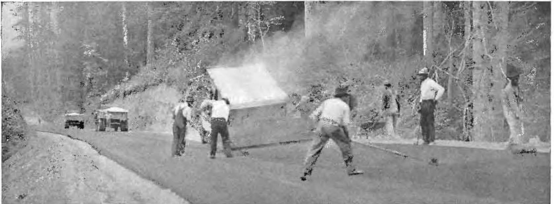
QUICK ACTION was obtained with the new mixture. A few rakers were used but the roller was able to follow close to the spreader instead of three to five hours behind as with regular mixes.
