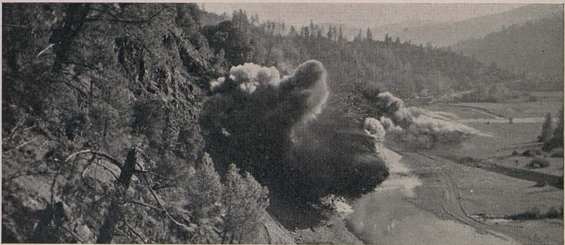
IT WENT BOOM and 10,250 yards of solid rock were torn from this bluff and hurled into the Trinity River.
