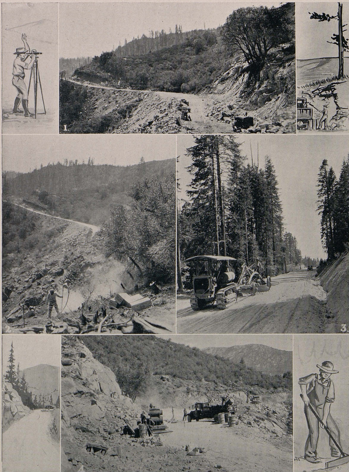
ROAD TO PARADISE for the lover of scenic grandeur would fittingly describe the Kings River Canyon Highway now under construction. No. 1 shows the present "end of the trail." No. 2, a blasting operation for new construction. No. 3, grading equipment at work. No. 4, unloading gasoline at "the front" for motor and camp use.
