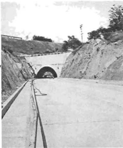
BROAD AND SMOOTH is the way now through the west portal of the Newcastle bore.
