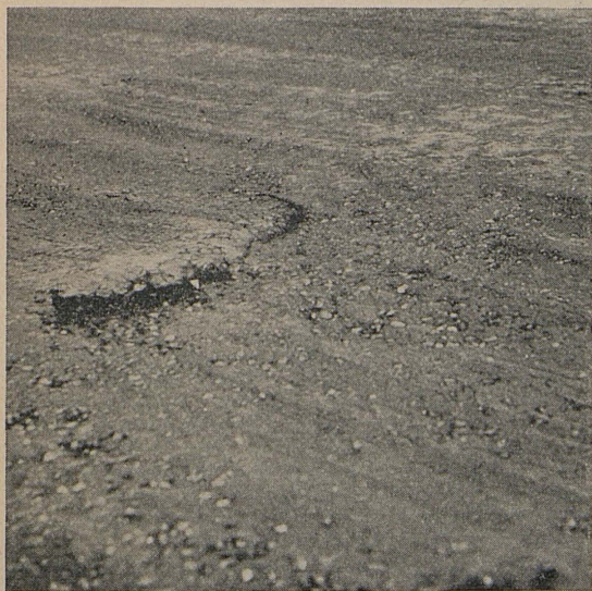
TOO MUCH OIL in the mixture causes the road surface to become pushed and rutted under traffic due to instability and resulting in much quicker deterioration with a largely increased expense for maintenance.
