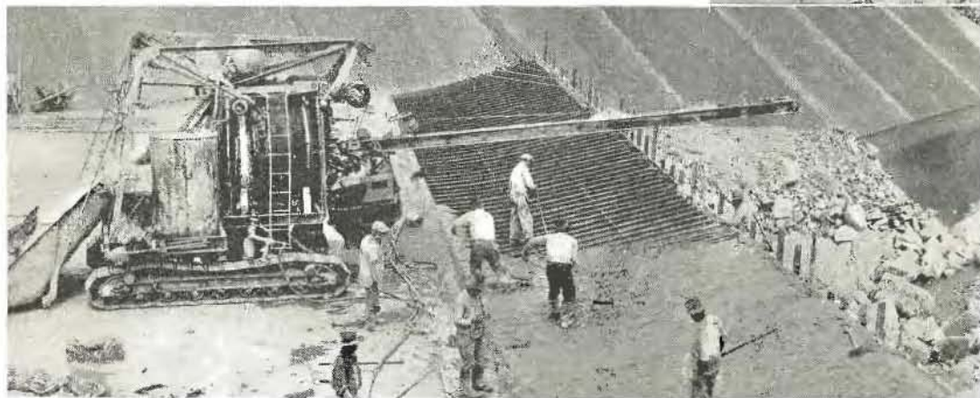
HERE SHE ZOOMS —Workmen are constructing a heavily reinforced concrete take-off at the outlet end of the concrete channel that will force the water to make an aerial leap of sixty feet to prevent undercutting. The "Zoom" has a 12\frac{1}{2} degree upward angle to a heavy cut-off wall.
