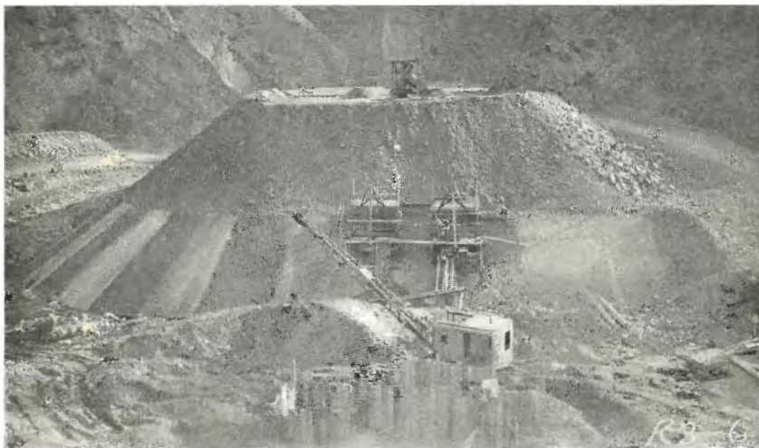
MASSIVE PREPARATIONS are here shown for a bridge in Piru Gorge. The slope of the huge fill is paved to protect the embankment and piers are being built through boxes extending down to the foundations.
