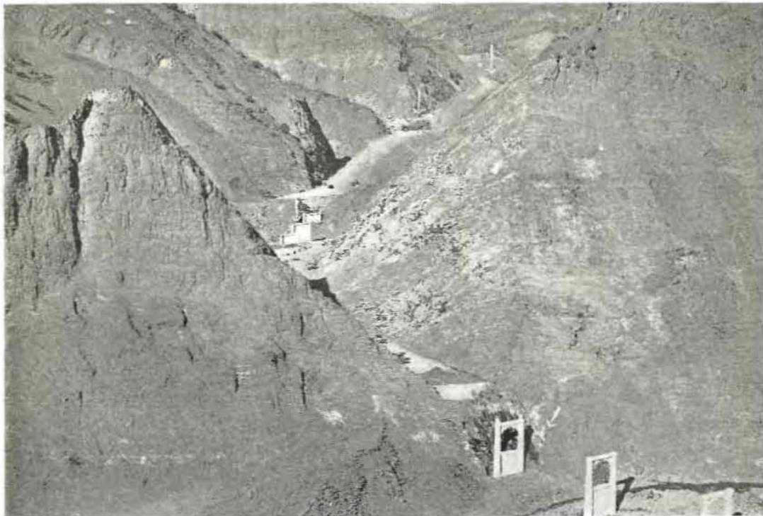
LIKE ORIENTAL SHRINES extending up the rugged canyon in groups these bridge piers looked when this photograph was made of the construction projects along the Ridge Route Alternate in Piru Gorge. Four bridge sites are visible in the picture as indicated by arrows.
