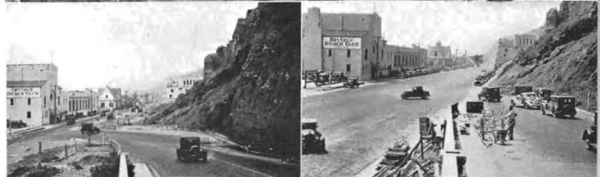
FROM BOTTLENECK TO BOULEVARD —Improved link of State Highway No. 60 at Santa Monica along the coast below the Palisades, now a fine four-lane highway is pictured at top. The old 20-foot pavement with the widening operation under way is shown in center picture, and below are “before” and “after” views of the California Avenue Incline connection.
