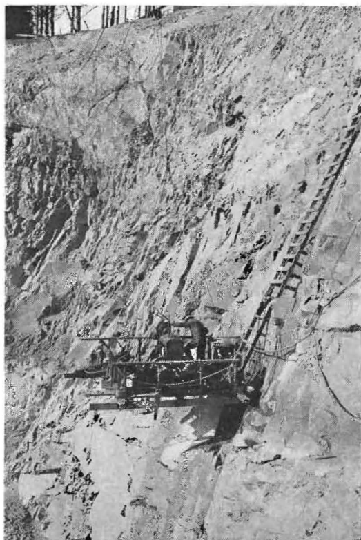
AN AIRY PERCH is provided for this equipment on the face of the west portal of the Yerba Buena Island tunnel where a 200-foot grout hole is being drilled.
