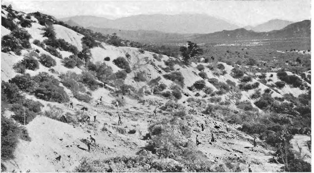
DESERT HILLS SHAVEN AND SHORN of shrubbery by unemployment relief quotas of highway workers mark the route of the Cajon-Lancaster link across the southern end of the Mojave Desert that will establish a new connection between northern and southern California via San Bernardino, Cajon Valley, Lancaster and Bakersfield. The clearing and grubbing is being done largely by hand labor.
