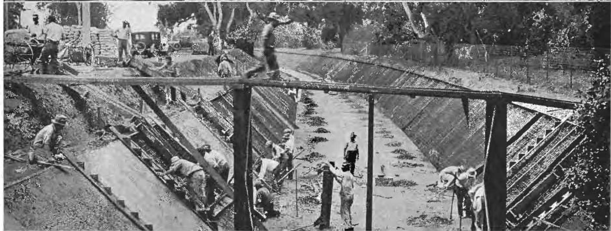
BUILDING TRUCK BY-PASS through the busy city of Santa Barbara. 1—Clearing operations for traffic separation structure. Note dangerous approach of old road to the underpass under railroad. 2—Grading operations near southerly city limits. 3—Constructing a reinforced concrete arch culvert at San Rocque Creek. 4—Paving side slopes of new channel for Mission Creek. It will have a 20-foot bottom and 9-foot depth.
