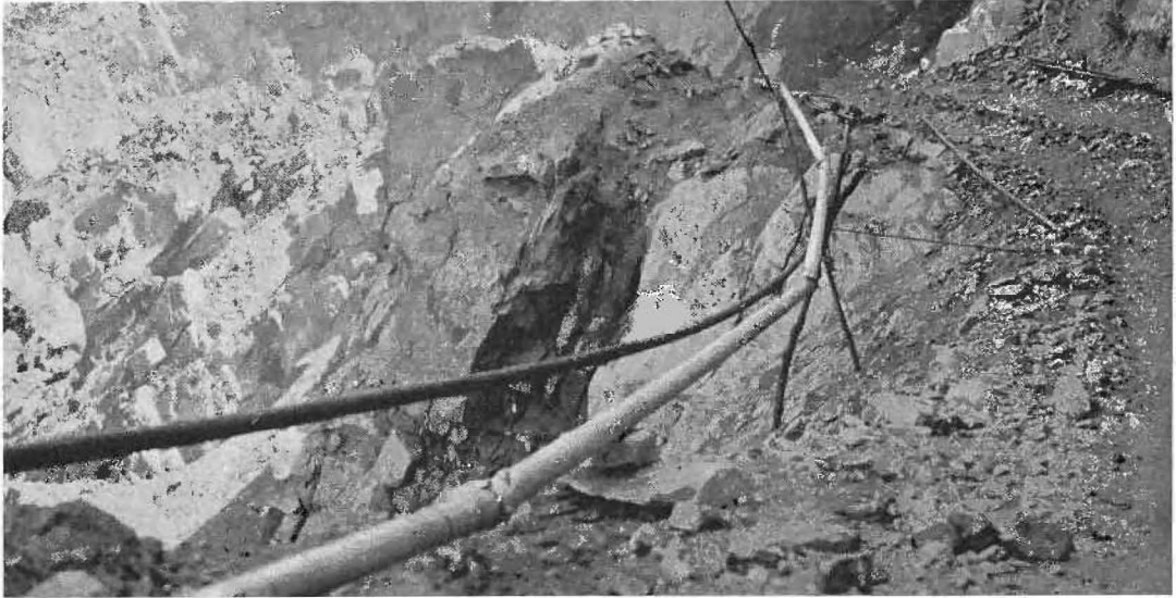
SPEEDY DRILLING is obtained on heavy rock work by the use of this light, large diameter, welded air pipe equipped with quick coupling device.
