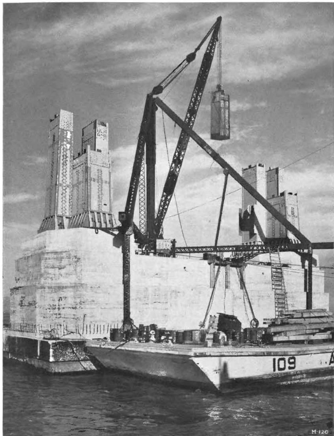
UP IN THE AIR goes segment after segment of Tower No. 2 of the San Francisco-Oakland Bay Bridge as great derricks swing aloft the huge crate-like steel units and pile them up like blocks on top of each other. As they are dropped into the place they were made to fit, riveting crews soon fasten them together. Thus the tower is rising slowly and steadily to equal the height of a 40-story building. Nine segments weighing a total of 1,500,000 pounds and towering 70 feet above the concrete base off the foot of Harrison Street, San Francisco, had been placed by March 17.
