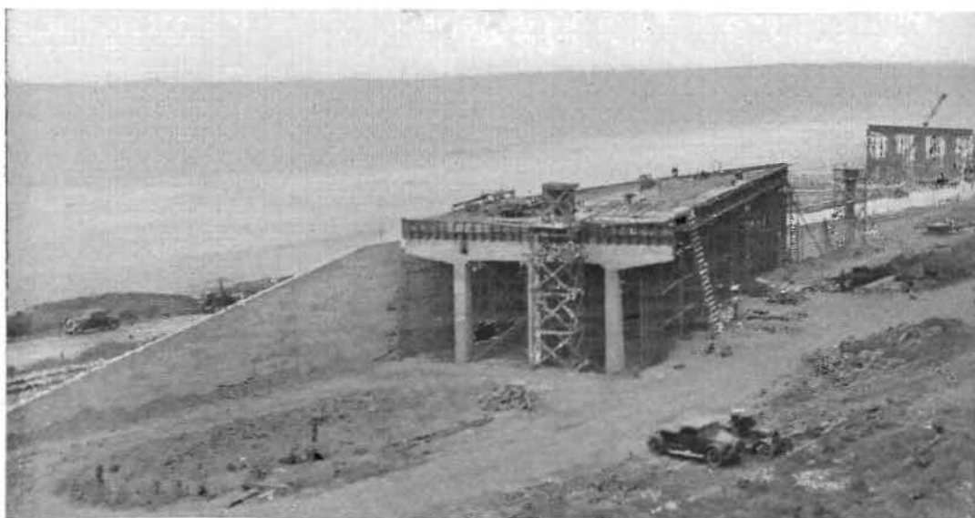
VENTURA OVERHEAD in course of construction. It will separate grades of railroad and highway.
