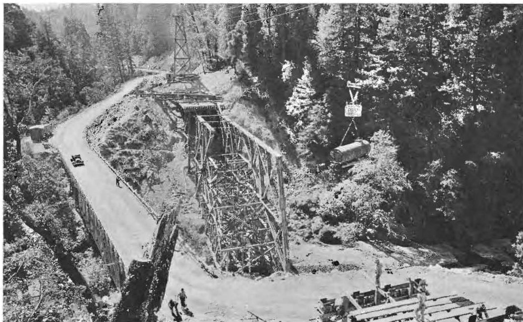
NOVEL BRIDGE DESIGN is incorporated in this structure over Rattlesnake Creek on the Redwood Highway in Mendocino County. Metal ring connectors are used in the center span. Truss spans were framed on the ground and lifted into place by a high-line.
