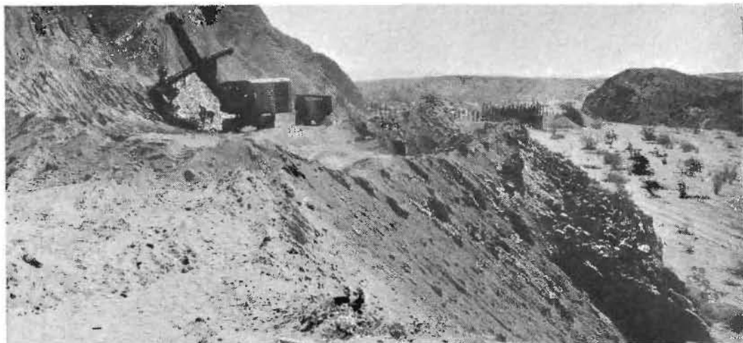
PIONEERING OPERATIONS are well advanced on the Indio Cut-off from Shaver's Wells on the Mecca-Blythe highway to State Highway 26 just south of Indio in Riverside County. The new road is being cut through desert hills as shown in the above picture. Preliminary construction for one of the bridges over a wash is seen in the background.
