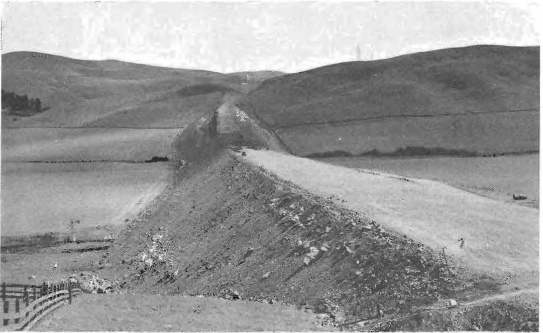
THE "BIG FILL" of the cut-off is rapidly growing to its designed proportions of 75 feet height and 2500 feet length with a width to accommodate a 40-foot pavement. Excess material from the Big Cut slides is being used to raise and widen the fill to its estimated volume of 605,600 cubic yards. In the center of the fill a timber and concrete bridge is being built.
