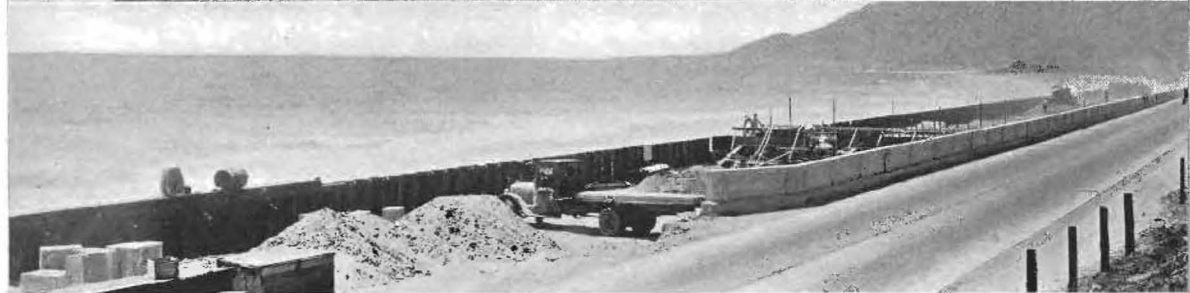
STEEL WALLS DEFY OCEAN'S power on the Coast Highway North of Ventura where a change of alignment, elimination of a dangerous underpass and widening operations compel the use of more ocean front right of way. The upper photos show the new overhead structure crossing the existing highway and swinging out on the beach with a portion of the protective steel sea wall already built. The central picture is a close-up of the interlocking sheet steel piling driven to elevation 10.0 feet held in line by the rods extending to concrete dead men. Below, general view of the 3,802 lineal feet of new seawall.
