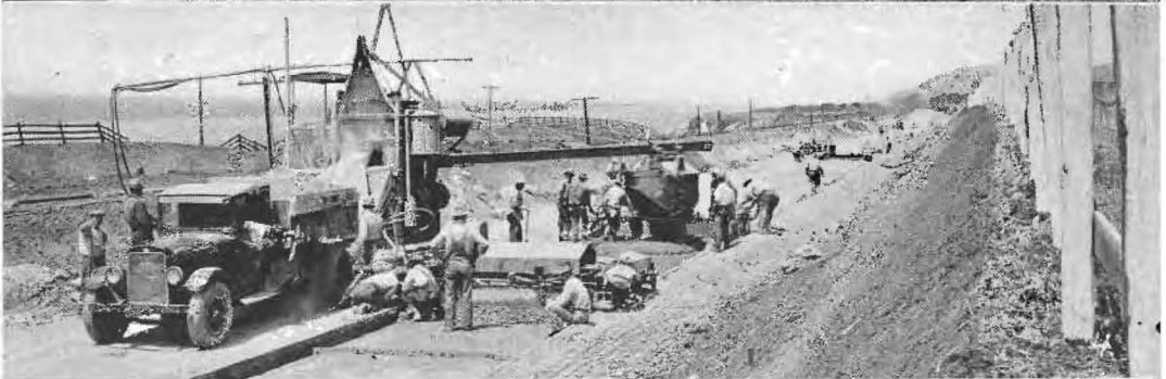
MODERNIZING THE COAST HIGHWAY between Arroyo Hondo and Gaviota in Santa Barbara County, the work of widening the roadway, realigning and removing dangerous dips and curves is about completed. No. 1 is a recently opened section of new highway. No. 2 view of big fill at north end of project looking toward Gaviota with rolling operations in progress. No. 3, fill under construction between railroad and old highway seen at left. No. 4, pouring concrete. Note two tamping machines at work, one for the base course on which to place wire mesh reinforcing and one for the surface course.
