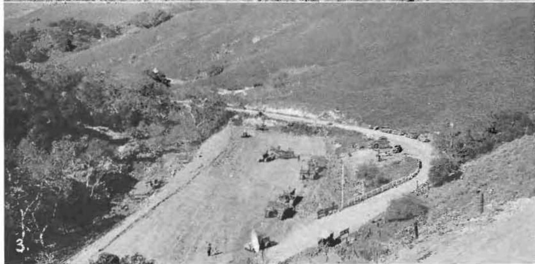
NOJOQUI GRADE REALIGNMENT of U. S. 101 through Gaviota Pass in Santa Barbara County involves some heavy grading, 581,000 cubic yards as shown in pictures 1 and 2 and elimination of 33 curves as in No. 3.
