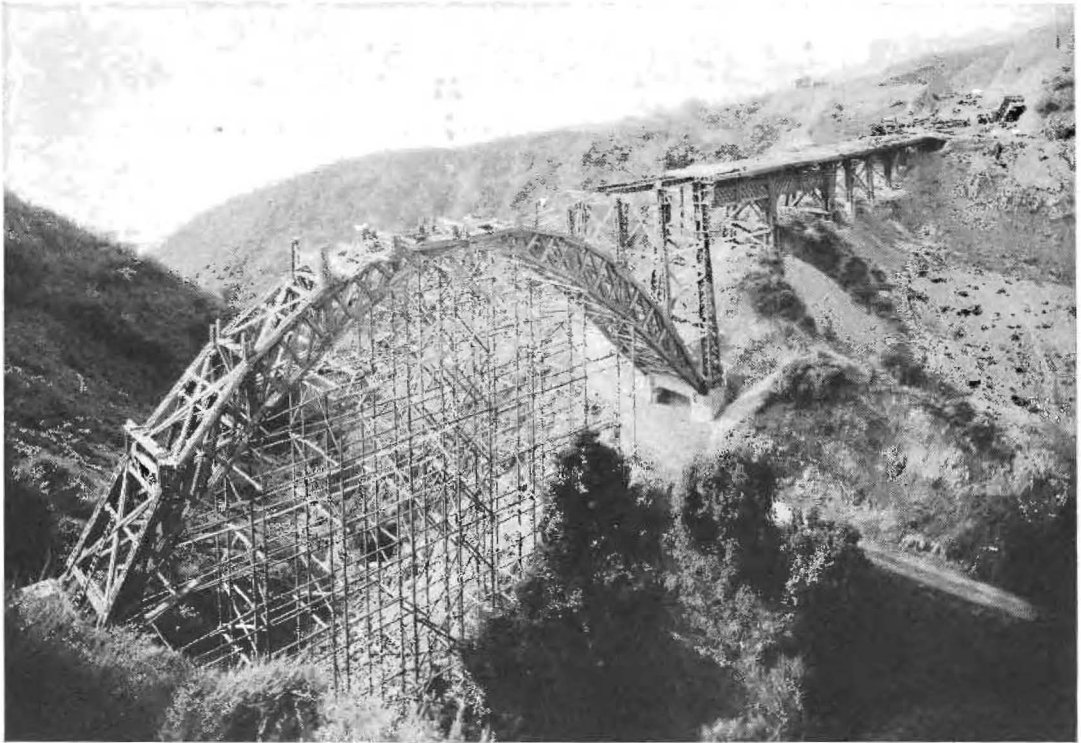
DOLAN CREEK TIMBER ARCH —This 180-foot span on Carmel-San Simeon highway involved some pioneering construction for a timber span of such length. Metal ring connectors were used to increase the strength of the timber joints.
