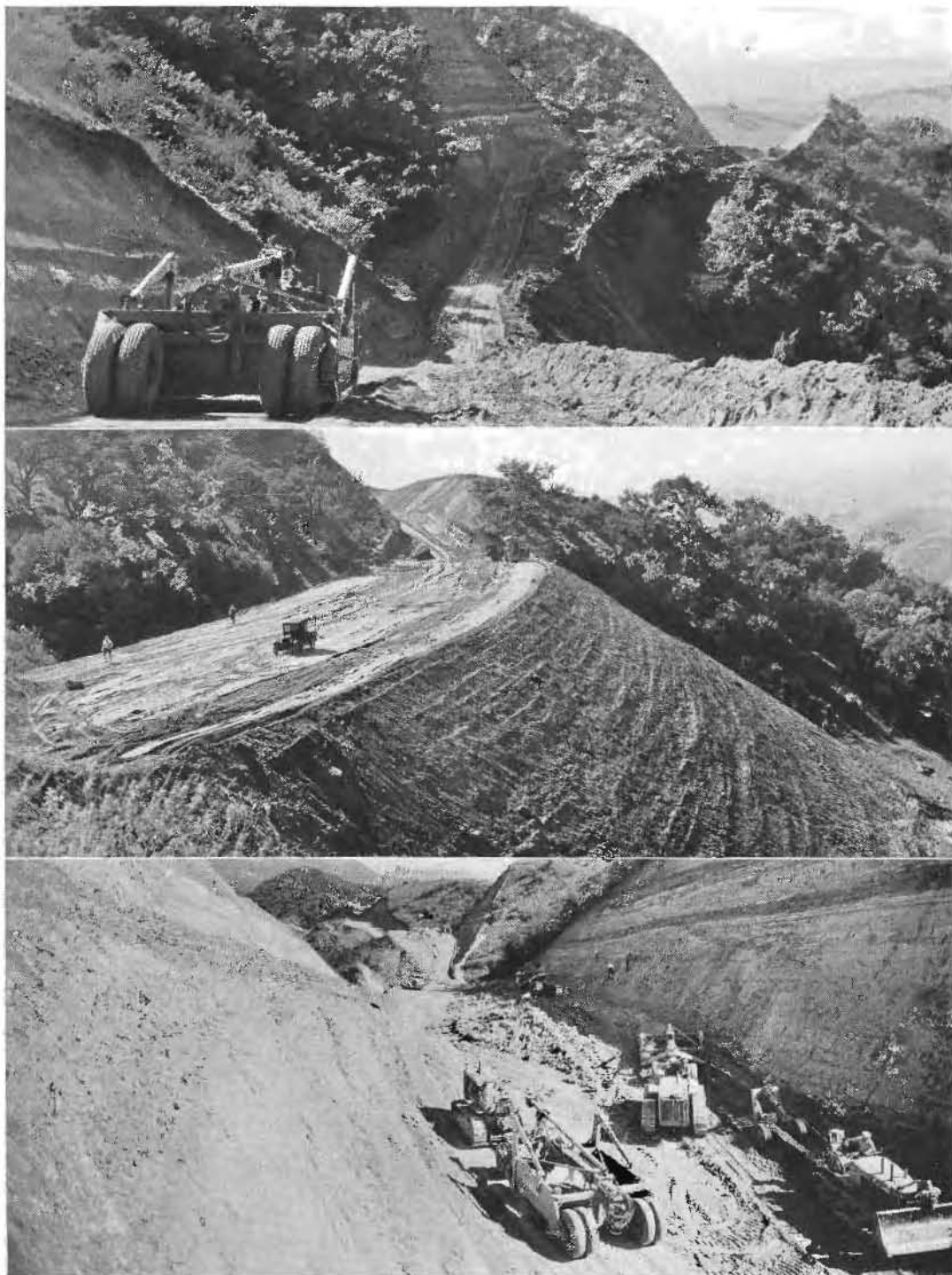
SAN MARCOS PASS CONSTRUCTION SCENES. At top a scraper is working on a preliminary fill leading to two 100-foot cuts seen in background. Center picture shows a 100,000 cubic yard fill nearing completion. The bottom view shows three scrapers and a 75 horsepower bulldozer in operation on one of the 100-foot cuts, illustrating the heavy grading work required on many portions of this rugged mountain terrain where a realignment of the existing steep and tortuous highway is now in progress.
