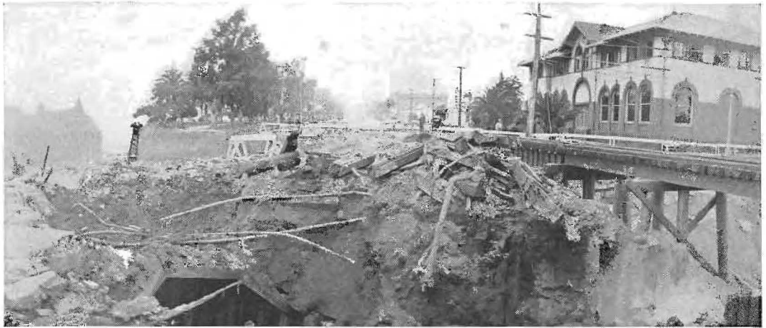
OPEN CUT CONSTRUCTION from the Beach road through Palisades Park and Ocean Avenue at Santa Monica to build tunnel for new highway. Part of old railroad tunnel shows in foreground.
