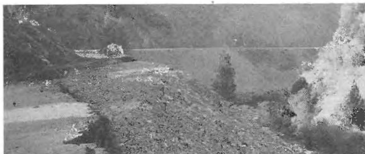
SLIP-OUT on the Feather River Canyon Highway on State Route 21 in Butte County.
