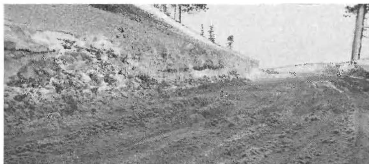
SURFACE FAILURE on State Highway No. 83 due to frost and heavy traffic.
