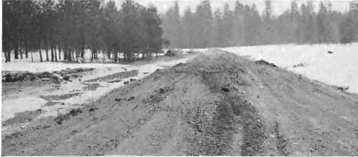
SURFACE BREAK west of Donner Summit caused by thawing and heavy trucking.
