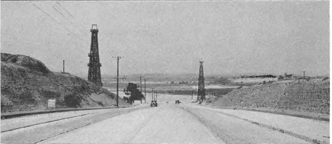
STATE STREET PROJECT extending between Redondo and Long Beach involved setting back power and oil lines to increase road width particularly through the Signal Hill oil district, where the roadway was narrow as shown in top picture. Below is a section of the new highway between Wilmington and Redondo—two 10-foot strips of concrete separated by a 20-foot strip of asphaltic concrete. Bottom picture shows a completed portion in the Signal Hill area widened to provide a six-lane arterial.
