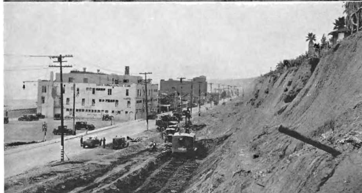
SANTA MONICA COAST HIGHWAY extension and widening operations—In the top picture workmen are constructing reinforced concrete slope protection for retaining walls that support walks and roadways on private property. Center picture shows a portion of the old Southern Pacific Railroad right of way through which the highway will be extended from the shoreline to Lincoln Boulevard by open cut and construction of a 400-foot reinforced concrete arch tunnel under Ocean Avenue and Colorado Avenue in Santa Monica. The tunnel will have a clear span of 56 feet and 48-foot roadway with sidewalks. In the lower picture steam shovel equipment is widening the right of way where the shoreline highway, at its lower end, starts to swing through the cut and tunnel and over Pennsylvania Avenue to the connection with Lincoln Boulevard.
