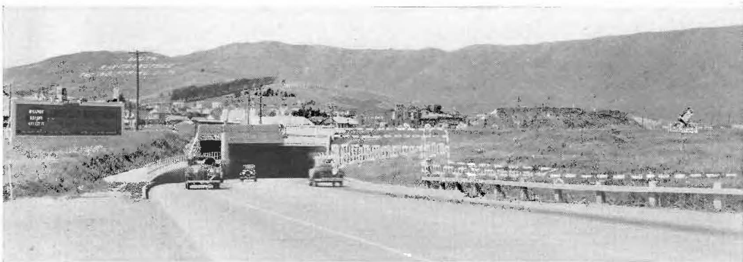
FORTY FEET MORE WIDTH of roadway will be provided through the underpass by extending the structure as shown by dotted lines on view of approach from north.
