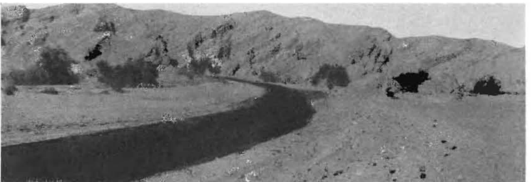
BEFORE AND AFTER THE FLOOD. The above pictures show two sections of the 7-mile stretch of highway in Box Canyon, Riverside County, that was entirely destroyed by a cloudburst storm on August 23d last and the restored highway as completely graded and surfaced on new location and better alignment and opened to traffic in 42 days.
