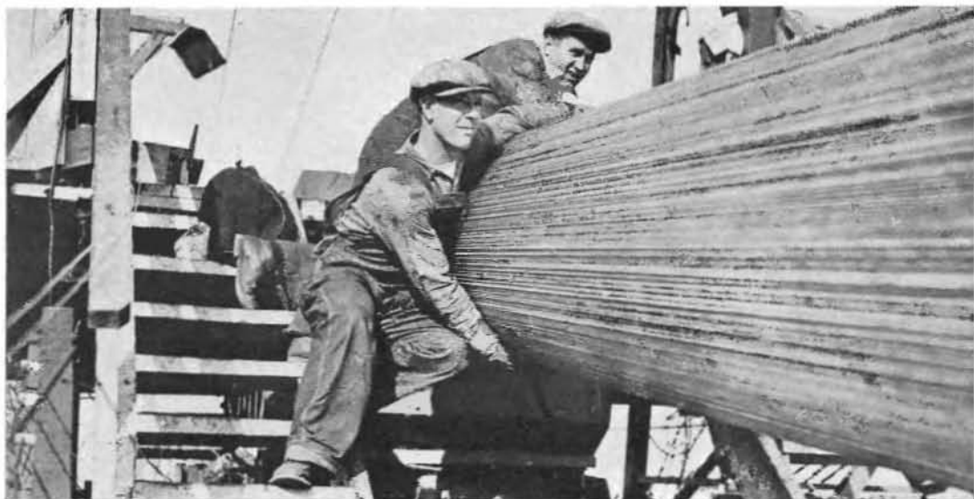
SO BIG! The two Bay Bridge workers are obligingly hugging one of the big cables to give an idea of its size before the compacting machine comes along and gives it a big squeeze. Photo courtesy of San Francisco Examiner.
