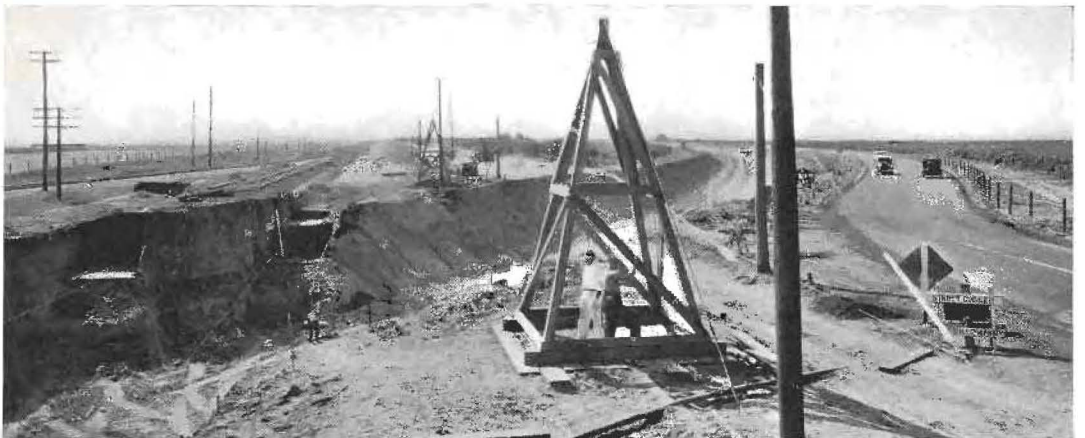
UNDER CONSTRUCTION. Both railroad and highway have been detoured to permit building of the Delano underpass. The new highway alignment, partially graded, is seen following along the cut embankment. Traffic is using the detour at right of picture.
