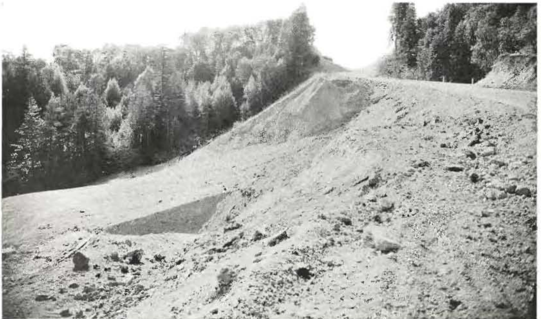
LOWER SLIDE AREA where 50 per cent of the fill slipped a distance of 300 feet down the mountain side and was stopped by trenching and backfilling with rock.
