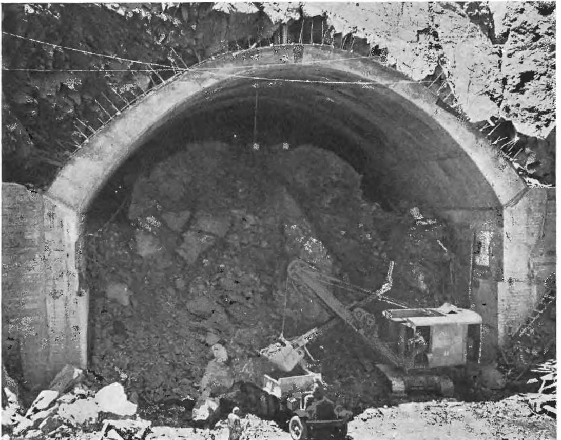
DOWN TO THE CORE. With the tunnel completely concreted and steel lined by novel construction methods a steam shovel begins removal of thousands of cubic yards of rock from 58 by 76-foot bore.
