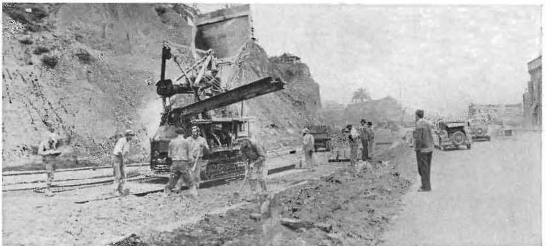
CONCRETE PAVER AT WORK on the widened Coast Highway along the Palisades in the Santa Monica beach recreational area in Los Angeles County. This contract provides a 76-foot pavement at a point of heavy traffic where the highway swings from the beach toward the portal of the Colorado Street tunnel now under construction.
