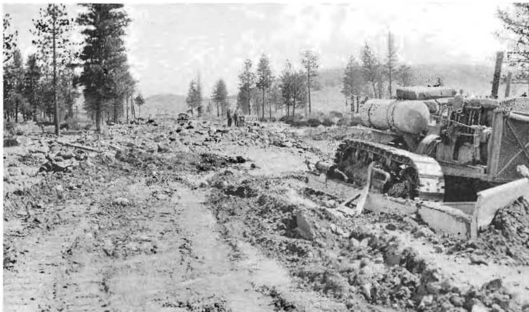
STATE HIGHWAY 72 BURIED under four feet of mud and boulders by flood waters from Mt. Shasta Glacier and Whitney Creek was cleared and opened to traffic in two days following the storm of August 28. The debris covered the road for a distance of 400 yards.
