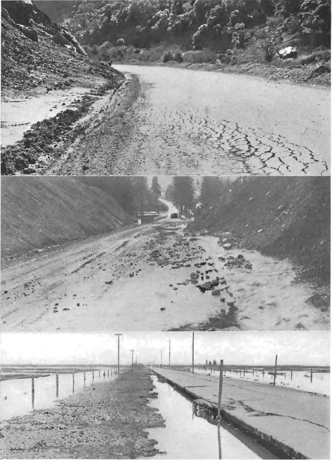
STORM DAMAGED HIGHWAYS. At top—Typical surface failure at mud slide on Coast Highway in Mendocino County. Center—Mountain stream diverted by blocked culvert wrecking highway. Bottom—Shoulder of Golden State Highway washed out by flood near Merced.
