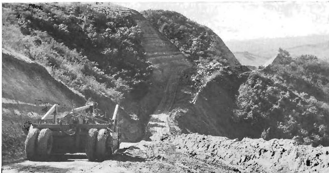
San Marcos Pass relocation construction presented much tough going for highway builders through rugged terrain of Santa Ynez Mountains.
