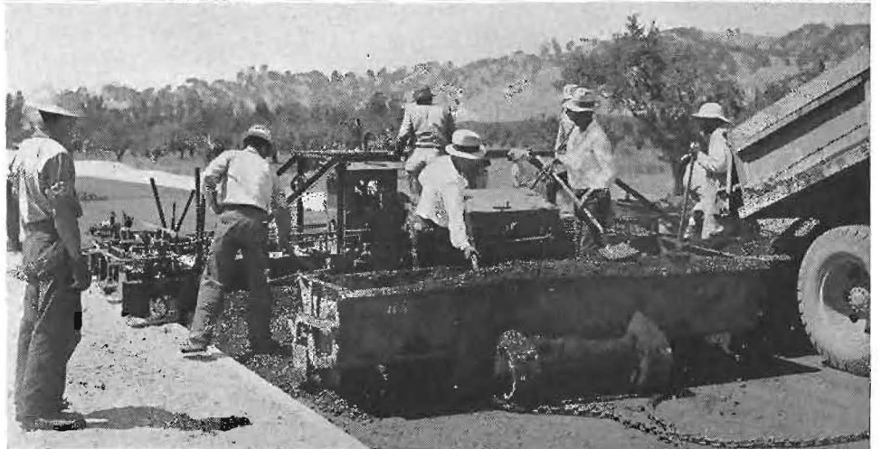
Busy scenes on the Fairfield-Vacaville relocation of U. S. 40 showing equipment placing 20-foot asphaltic concrete pavement. At top, trucks dumping into spreader boxes and mechanical finishing machine in operation. Center, equipment rolling finishing course. At bottom, close-up of spreader box finishing machine.
