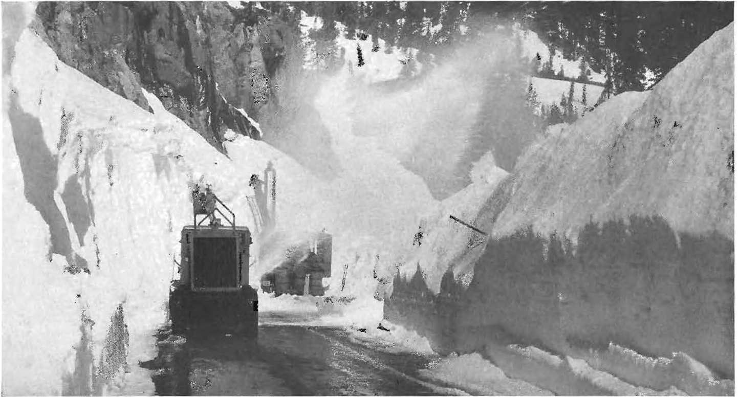
With average total annual snowfall on some highways exceeding 600 inches, snow removal is a big problem in Washington as shown in this photo of highway crew at winter work.
