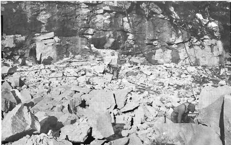
Building a highway along the face of a sheer cliff in Washington state.
