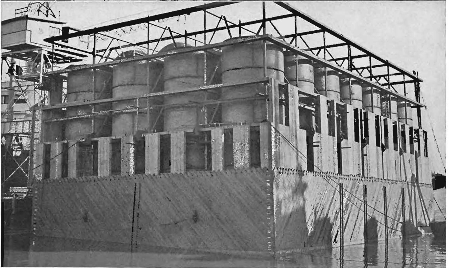
Views of flotation cylinder caissons used for the first time in bridge construction to build foundations for towers and central anchorage of San Francisco-Oakland Bay Bridge, which were shown on screen to delegates to convention of American Association of State Highway Officials by C. E. Andrew, Bridge Engineer. Upper—Showing how one caisson looked before pouring of concrete into steel tubes for sealing was completed. Inset—Air-tight domes on tubes through which air was pumped into cylinders, displacing the water, to make each cylinder act as air buoy until bottom of caisson rested upon rock. Lower—View of caisson from water level during sinking of cylinders.
