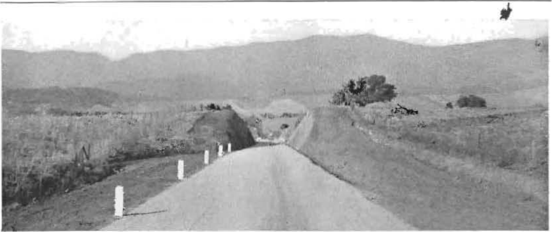
SAN MARCOS PASS highway just completed on new alignment over the Santa Ynez mountains.
