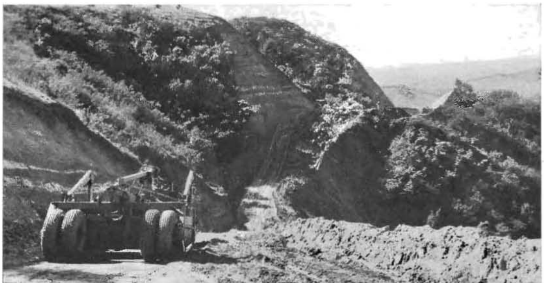
CONSTRUCTION SCENE showing character of heavy grading work on fill leading to two 100 foot cuts.
