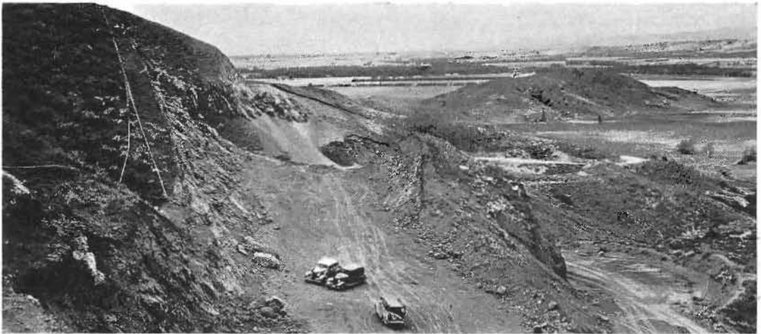
LARGE CUTS AND FILLS on new direct alignment; old winding road at right.
