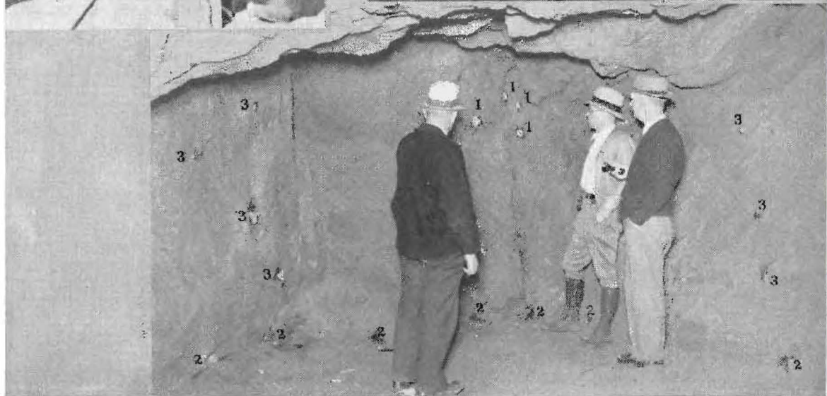
FEATHER RIVER TUNNEL BLAST scenes when bore No. 3 was holed through May 7th. Top picture, left to right, shows District Equipment Superintendent Siebert, Superintendent Rawson and Resident Engineer Webb being greeted by Superintendent Waste, Assistant District Construction Engineer, Lowden and State Highway Construction Engineer Pope as they crawled through hole after blast. Center—Mr. Pope setting off blast and cloud of smoke and debris caused by explosion. Bottom—Dynamite charges in heading ready to fire showing: 1—Breast holes; 2—Lifters; 3—Cut holes.
