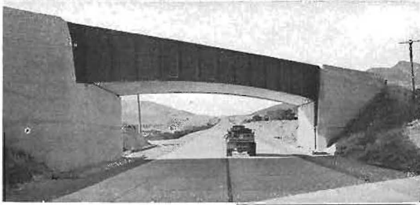
Above is Cordelia underpass and on right, view of big fill on cut-off
