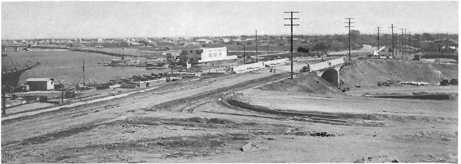
Two bridges and a system of four spacious ramp connections feature the extensive construction project separating the grades of the primary shows grading for the east ramp to the 3150 foot overhead alignment, and the new bridges over Coast Highway and Newport Channel. A
