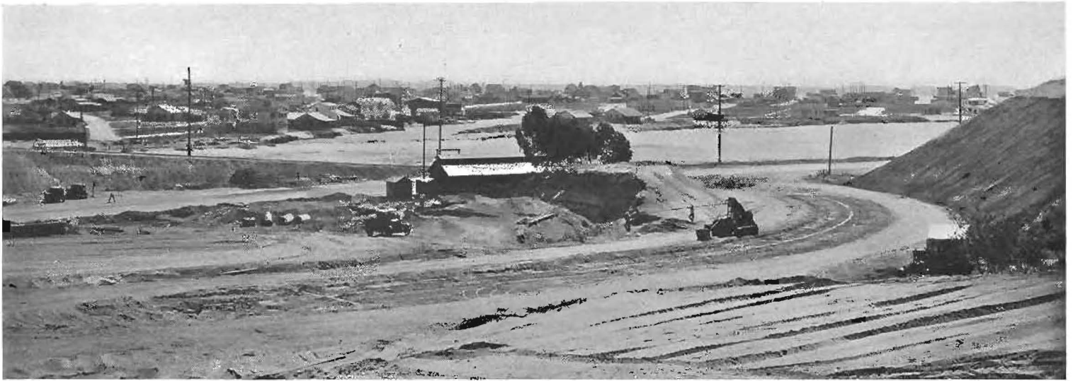
Coast Highway and the secondary Santa Ana-Newport Highway at Newport Beach, a badly congested intersection. This construction scene white arrow marks location of latter bridge which is 200 feet long and has a movable span to comply with Federal navigation regulations.
