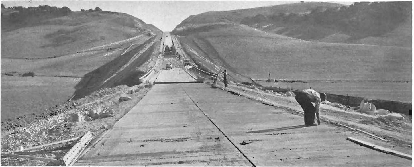
The "Big Fill" of the American Canyon Cut-off showing paving operations under way placing a 20-foot concrete surface.
