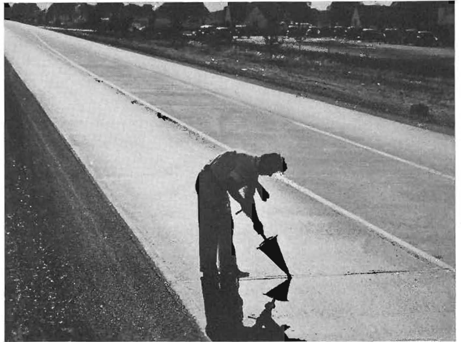
Placing improved filler by hand method at combined cost for labor and material of 65 cents per joint.
