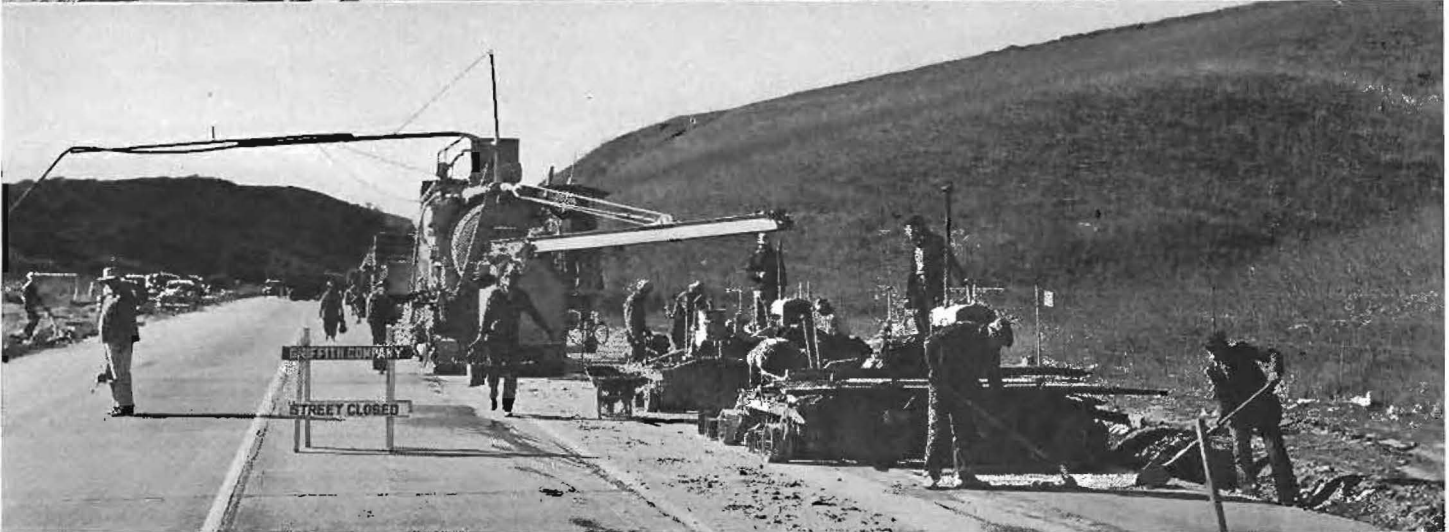
Views of realigned Los Angeles-Pomona Lateral, unusual airline highway, which provides a 27-mile stretch of road with only two "Stop and Go" signals and only two boulevard "Stop" signs for its entire length. Upper: Completed section of 40-foot pavement, widened from three to four lanes, west of Pomona. Center: Shows line of trucks dumping material used in laying additional 5-foot strip of pavement at left of roadway. Lower: Concrete mixer and mechanical finishers operating on Garvey Boulevard near Kellogg Hills one of links in new highway which will be completed in May. This project entailed the construction of a 10-foot widening strip and 8-foot plant mixed shoulders for a distance of 18.7 miles.
