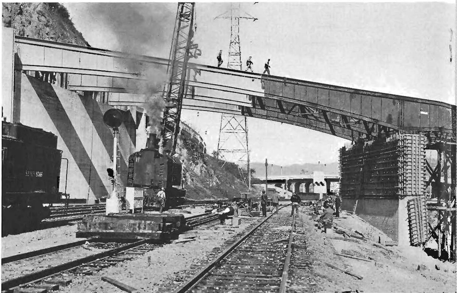
Center span is 200 feet long, one of the largest plate girder spans in the country. The other steel spans are 104 and 122 feet long.
