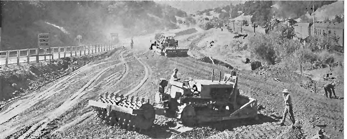
New Cuesta Grade in the making. Upper—Trucks excavating Summit Cut and hauling material down existing highway to fill north approach of overhead crossing Southern Pacific tracks. Center—Two tractors and master bulldozers and a roller pioneering one of fills. Lower—Leveling and compacting fill at north approach to proposed overhead crossing.
