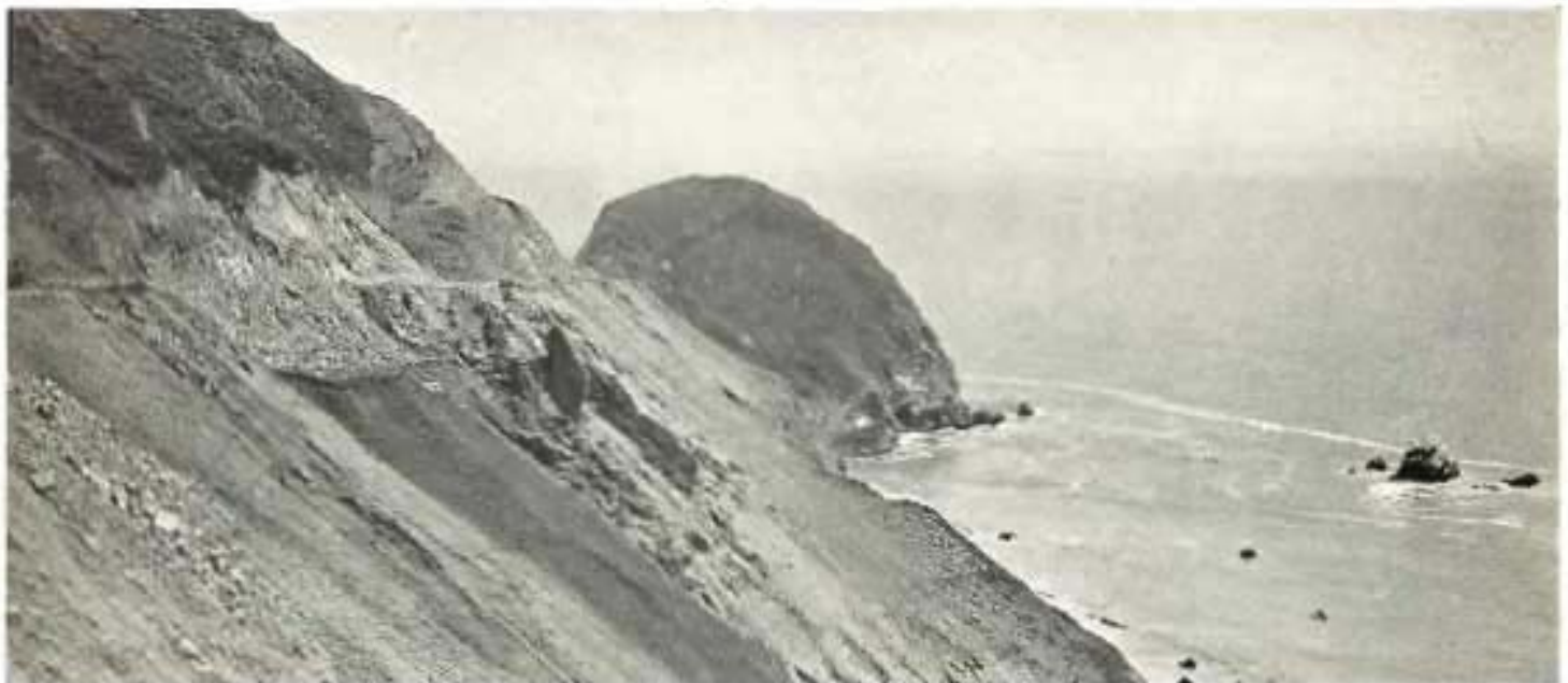
This picture vividly illustrates difficult construction on Ocean Shore Highway on Pedro Mountain.
