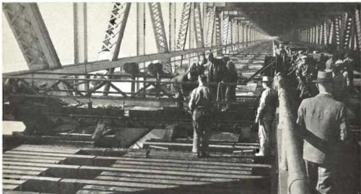
This picture shows the laying of ties for the San Francisco-Oakland Bay Bridge railway system at easterly edge of span.
