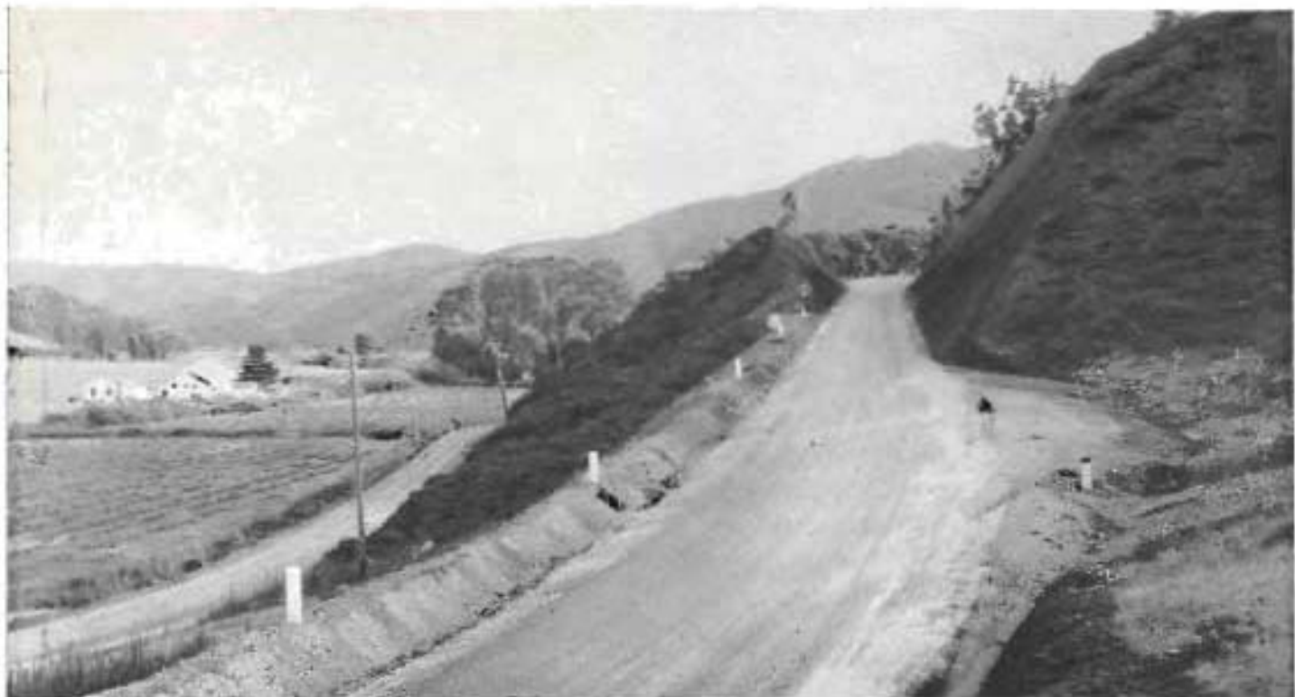
View of Ocean Shore Highway 1\frac{1}{2} miles south of Rockaway Beach. The old county road is shown on left.
