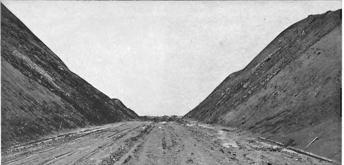
Scenes on the Vacaville realignment project, an improvement to a unit of State highway (U. S. 40) between Sacramento and San Francisco, by-passing the narrow and crooked streets of a congested section of the city of Vacaville. At top, new bridge and end of completed pavement where existing highway enters city on a curve. New alignment, rough graded, extends in direct line to connection with highway one-half mile east of city. Center, left, narrow bridge and street passing two schoolhouses, and at right, short radius "S" curves, schoolhouse in background. At bottom, a large cut on the new alignment.
