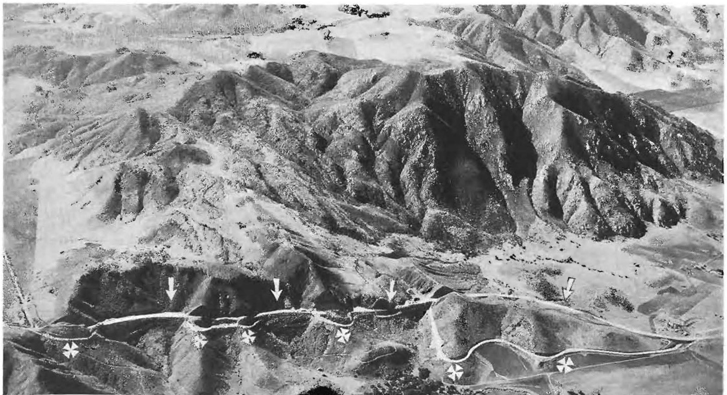
Broadside aerial view shows how new Conejo Grade eliminates curves on highway between Conejo Summit, extreme left, and Conejo Creek, extreme right. The new route pursues a straight course down through the hills by means of cuts and fills. The new route is indicated by arrows. Curves eliminated are marked by crosses. Photograph by Fairchild Aerial Surveys, Inc.
