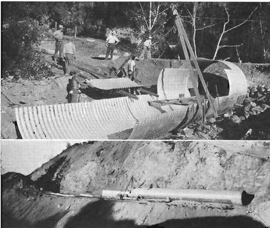
Upper photo shows size of multi-plate culvert used in construction of Carmel-San Simeon Highway. Lower—Long length of multi-plate culvert used 45 miles north of San Simeon on new road.
