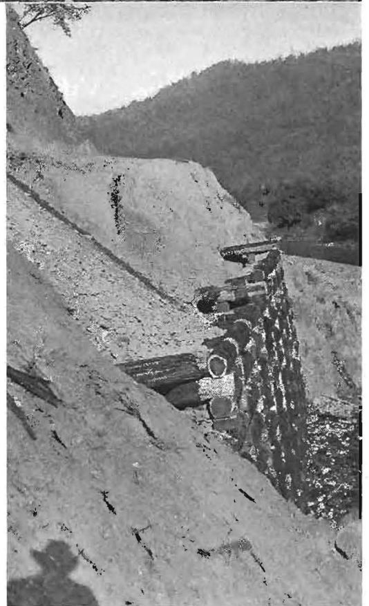
Upper picture shows size of Redwood crib on Trinity River to protect highway. Lower—View of river bed and road above where erosion occurred.
