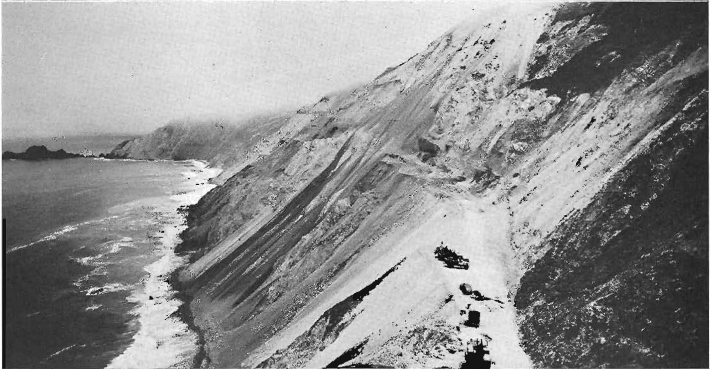
Scenes on Ocean Shore State Highway in San Mateo County now being built. Upper—Section of scenic route which will become modern highway. Center—Stretch of new highway with San Pedro Mountain in distance. Lower—Constructing highway along face of cliff on which engineers constantly battle slides which plunge into Pacific ocean below.
