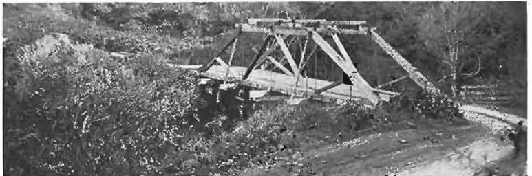
This 40-year old bridge over Elk Creek, Mendocino, has been cause of several severe accidents.
