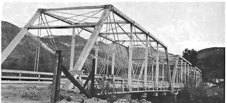
Type of combination truss span across Cottonwood Creek, San Diego, that is dangerous because roadway is too narrow.
