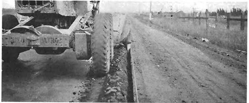
Disc attachment cuts compacted earth shoulders before placing plant-mixed surface on road.
