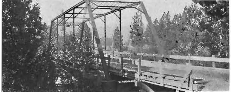
This bridge near Blairsden, Plumas, can be knocked down if hit by truck.
