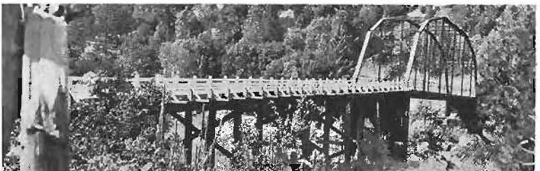
Klamath River bridge, near Seiad, Siskiyou, could not withstand blow from truck or auto.
