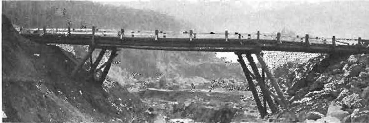
Oregon Gulch timber bridge, Trinity County, not safe for legal loads.
