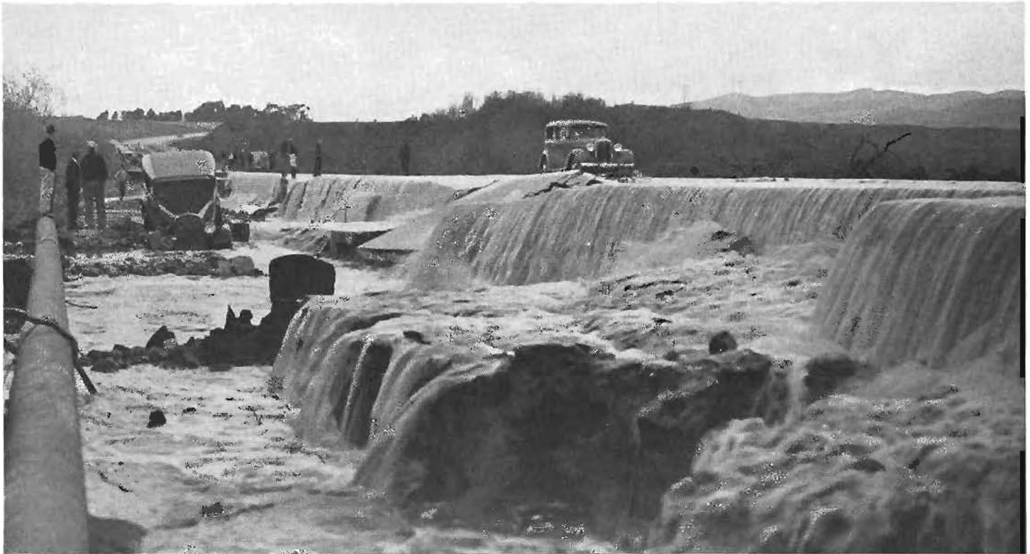
San Mateo Creek becomes miniature Niagara 20 miles north of Oceanside, San Diego County, and washes away highway pavement and shoulders.
