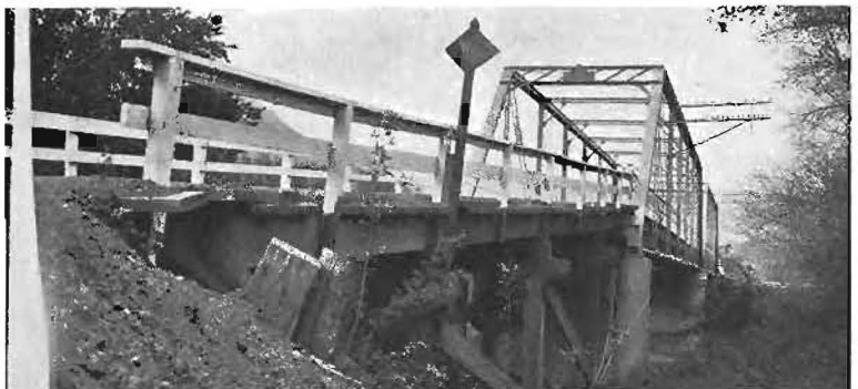
Dangerous structure with narrow roadway near Hopland, Mendocino.
