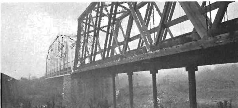
Supports under this timber truss on Yager Creek, Humboldt, wash out every year.
