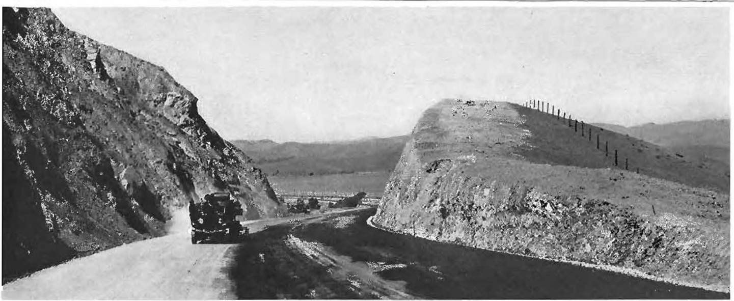
Waldo Approach looking down grade toward Richardson's Bay and junction of new road with State Highway at Waldo Point.
