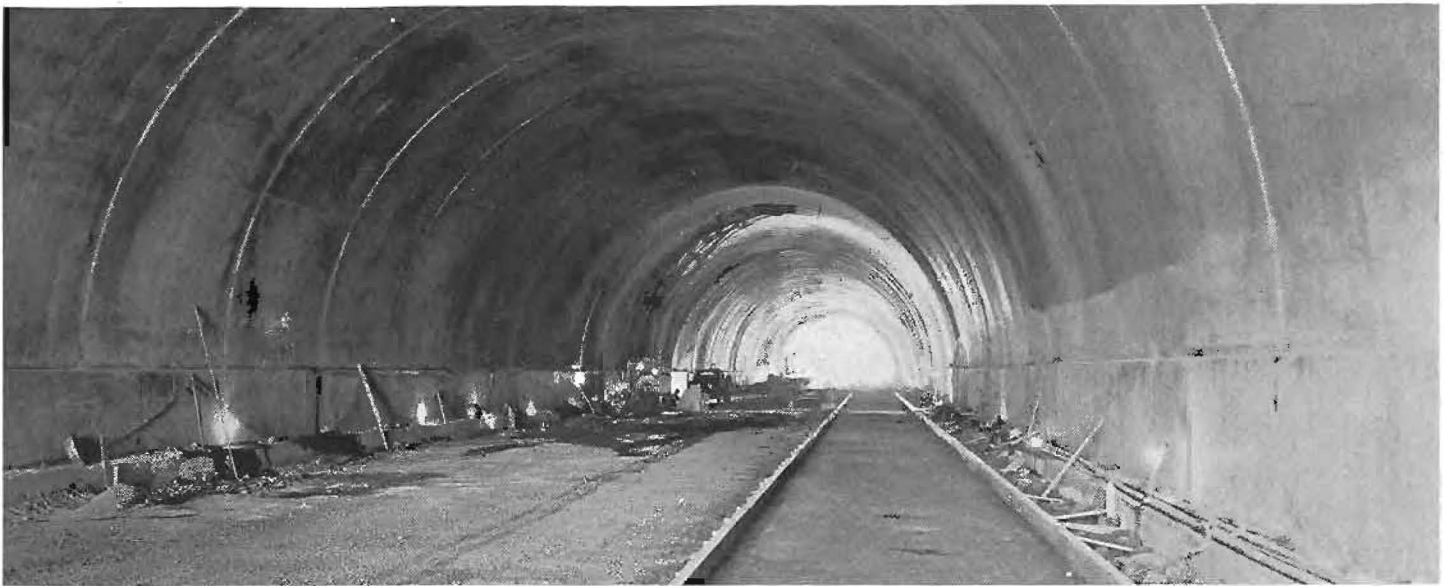
Interior view of State-built tunnel on mountain stretch of Marin approach to Golden Gate Bridge.
