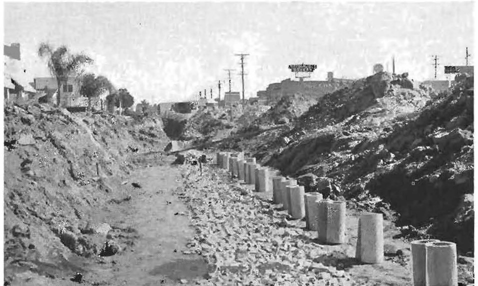
Approximately $340,000 was spent in providing proper drainage under and along three miles of El Cajon Boulevard. This picture was taken during construction.
