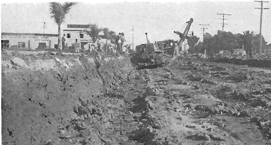
This picture was taken during excavation of unsuitable subgrade soil and abandoned pipe lines on El Cajon Boulevard.
