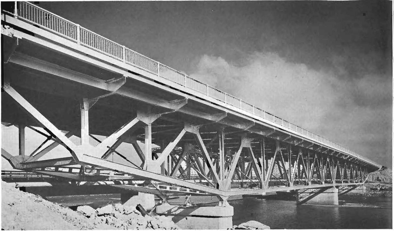
Recently completed steel and concrete bridge over Santa Margarita River with railroad bridge in background.
