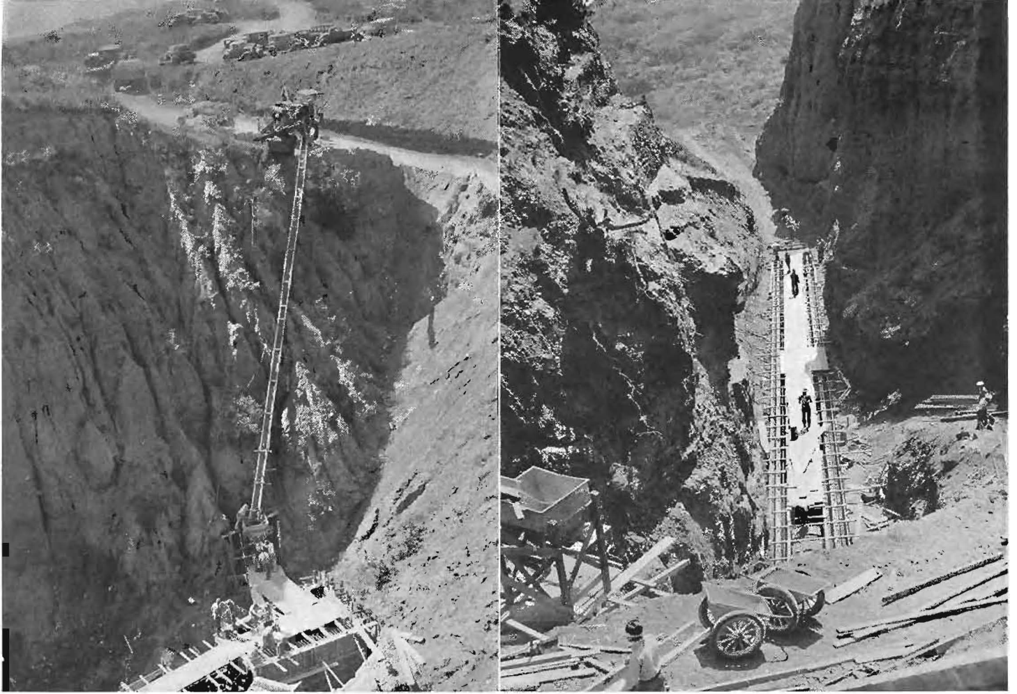
These pictures illustrate magnitude of highway culvert drainage construction on project north of Oceanside.
