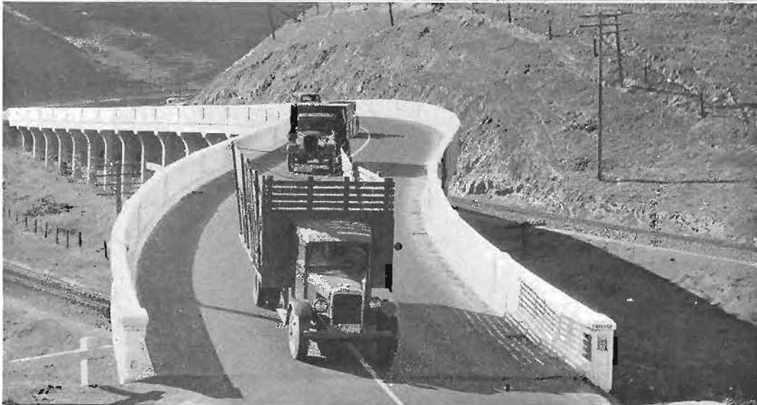
When new Altamont Pass Highway shown under construction in upper picture is completed there will be no traffic delays such as that shown in center picture and no traffic violations and hazards such as depicted on narrow Altamont bridge pictured below.
