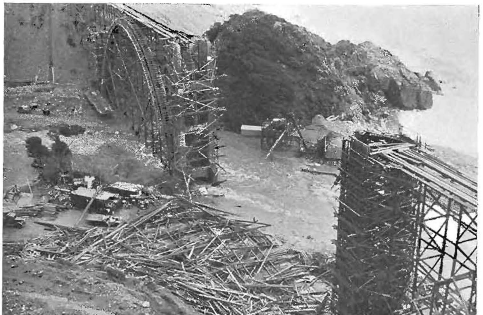
Bridge under construction across Big Creek on the San Simeon-Carmel coast highway in Monterey County. Concrete piers withstood flood waters but high winds blew down falsework of one arch.
