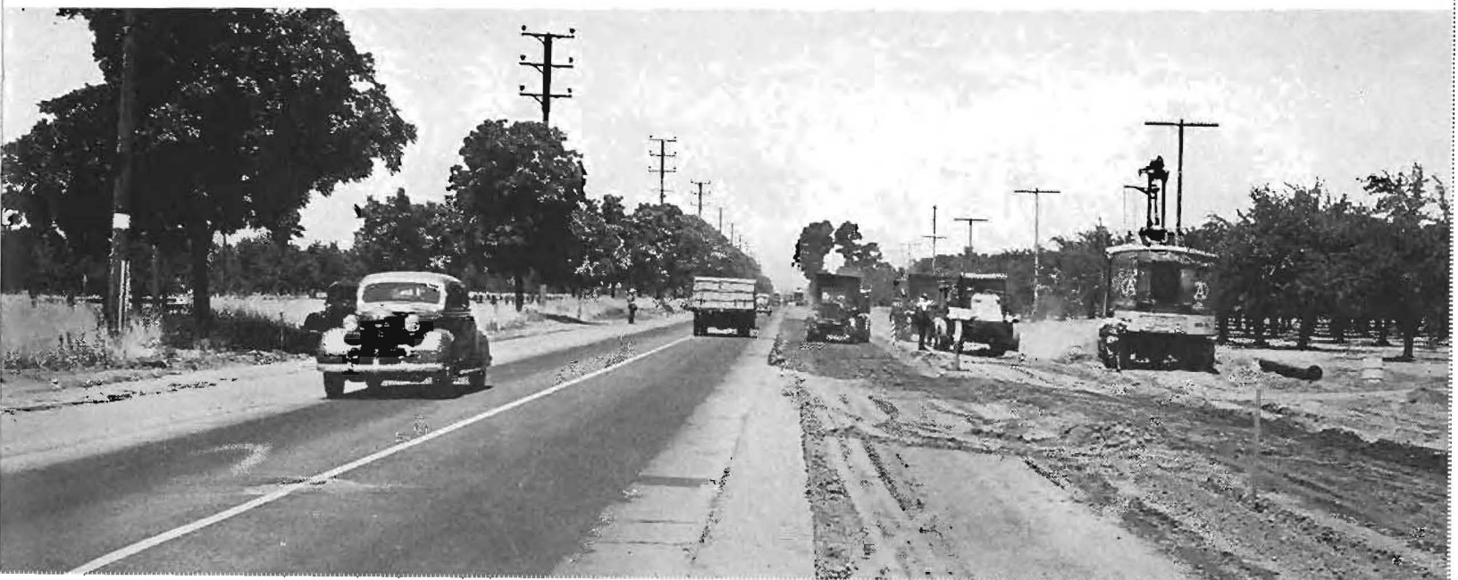
Shovel removing surplus excavation while trucks are placing borrow material along newly widened section of roadway.
