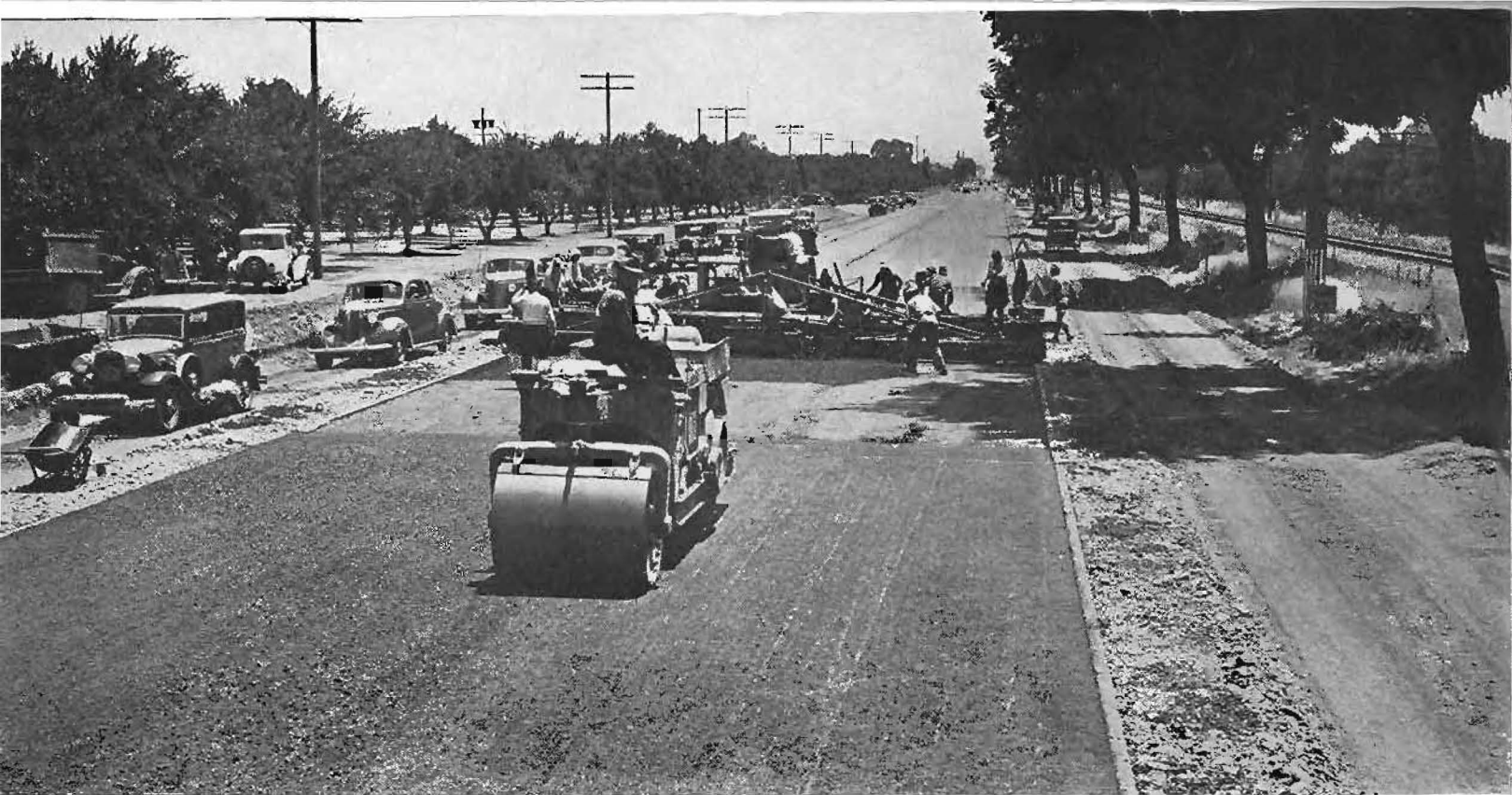
Thirty-three foot finishing machine spreading leveling course at end of asphalt concrete surface run on State Highway 101.
