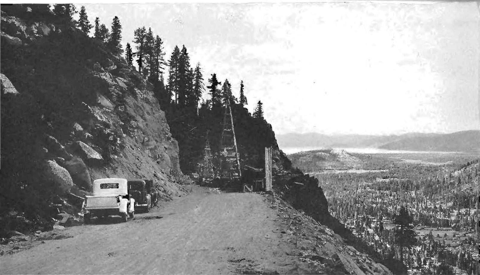
Partially completed highway relocation on east side of Echo Summit. Meyers in center right and Lake Tahoe in distance.
