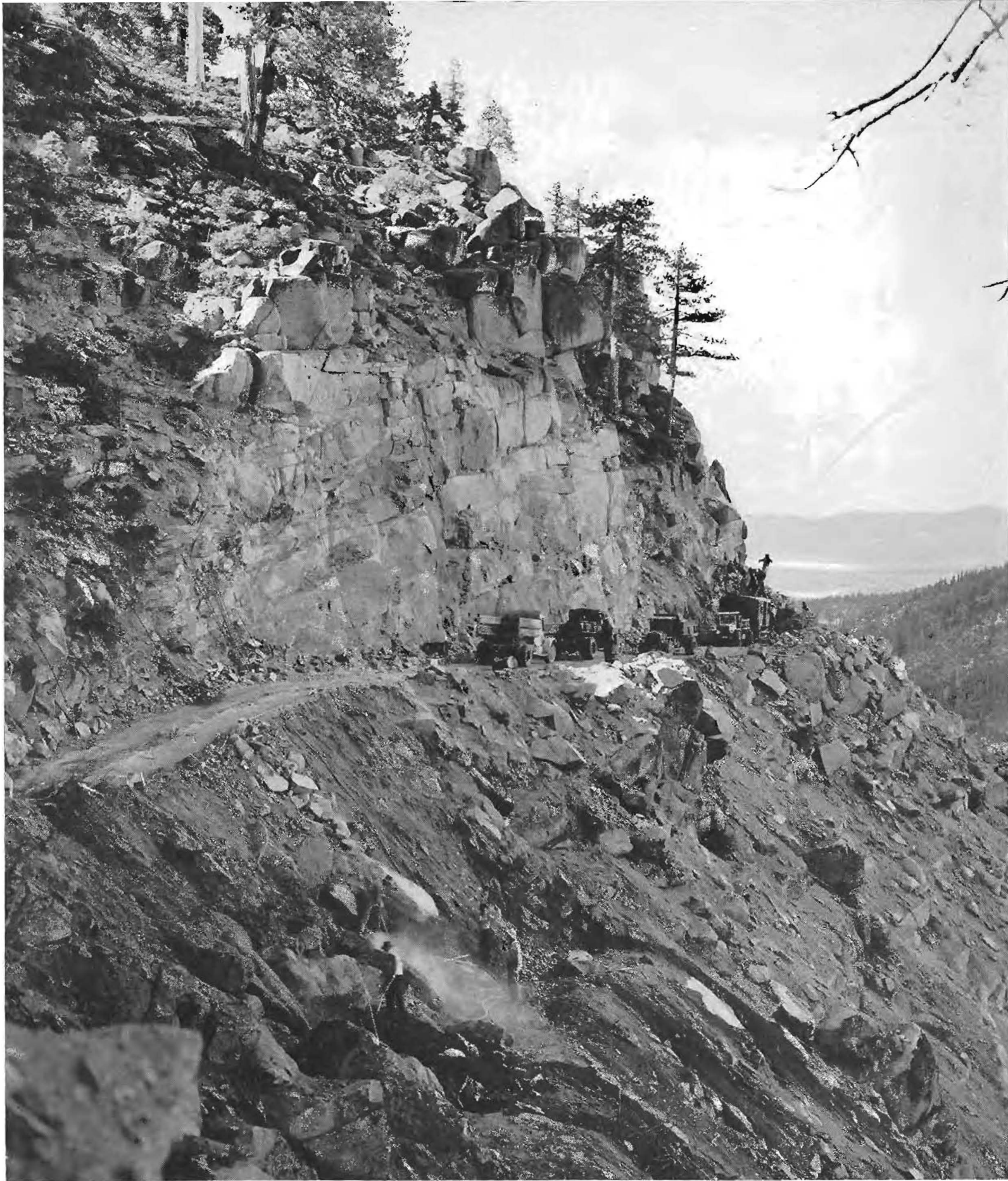
On sheer eastern cliffs of Echo Summit power shovel is making final cut for Meyers grade relocation. Lake Tahoe in distance.
