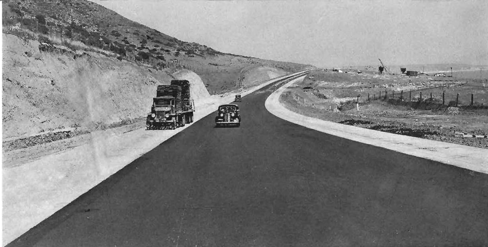
Division strip on this section will be 4-foot wide with raised white arrows bordered by double white lines.
