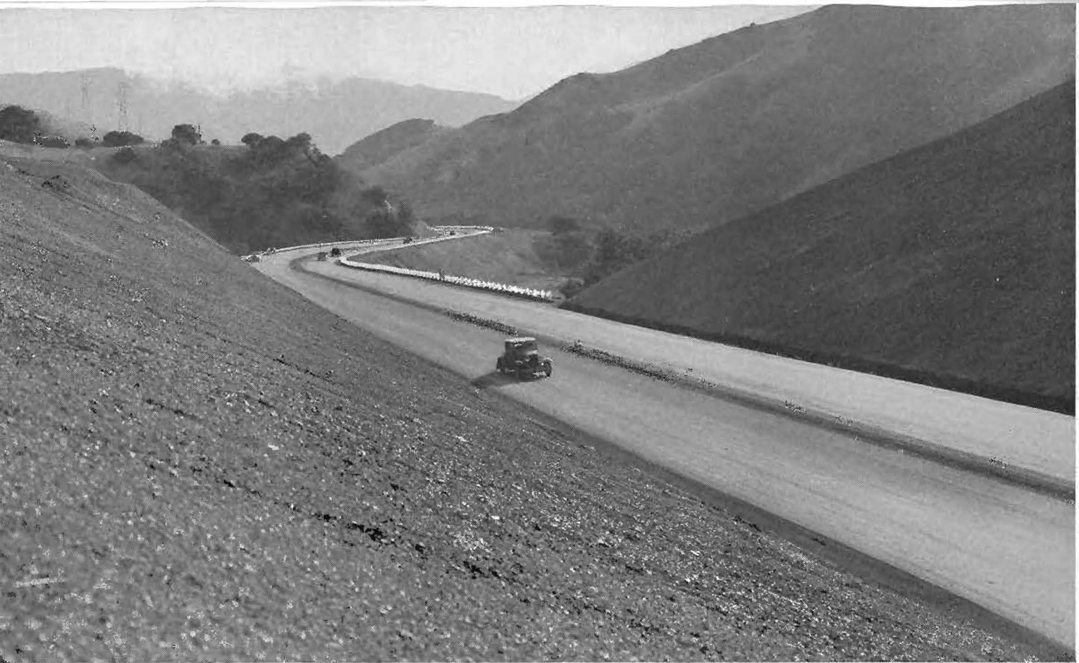
Section of new four-lane divided highway through Cuesta Pass. Center parting strip is unfinished and traffic striping yet to be done.
