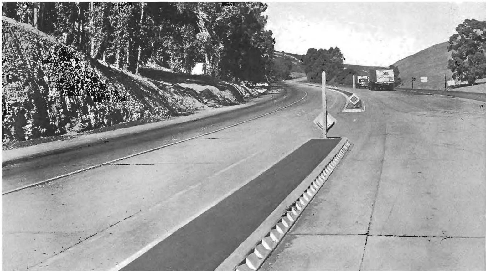
Curbing of center dividing strip has recessed panels painted to reflect light at night as an added safety design.
