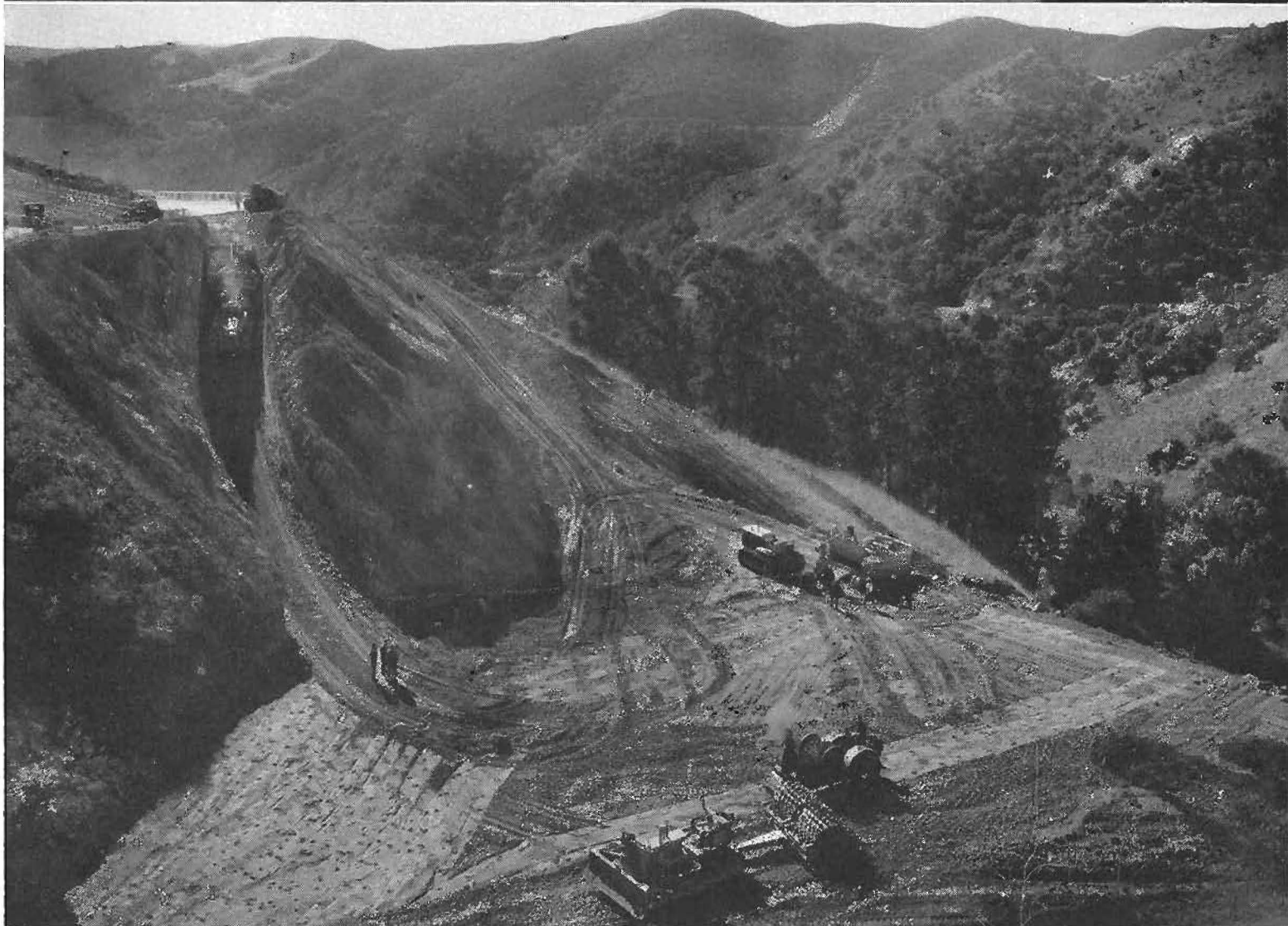
Top view shows wide roadbed and easy grade of new Cuesta Pass Highway providing 4 plant-mix surfaced traffic lanes separated by 4-foot dividing strip as yet unfinished and unstriped. At bottom, construction scene on huge fill that required moving 122,000 cubic yards of dirt.
