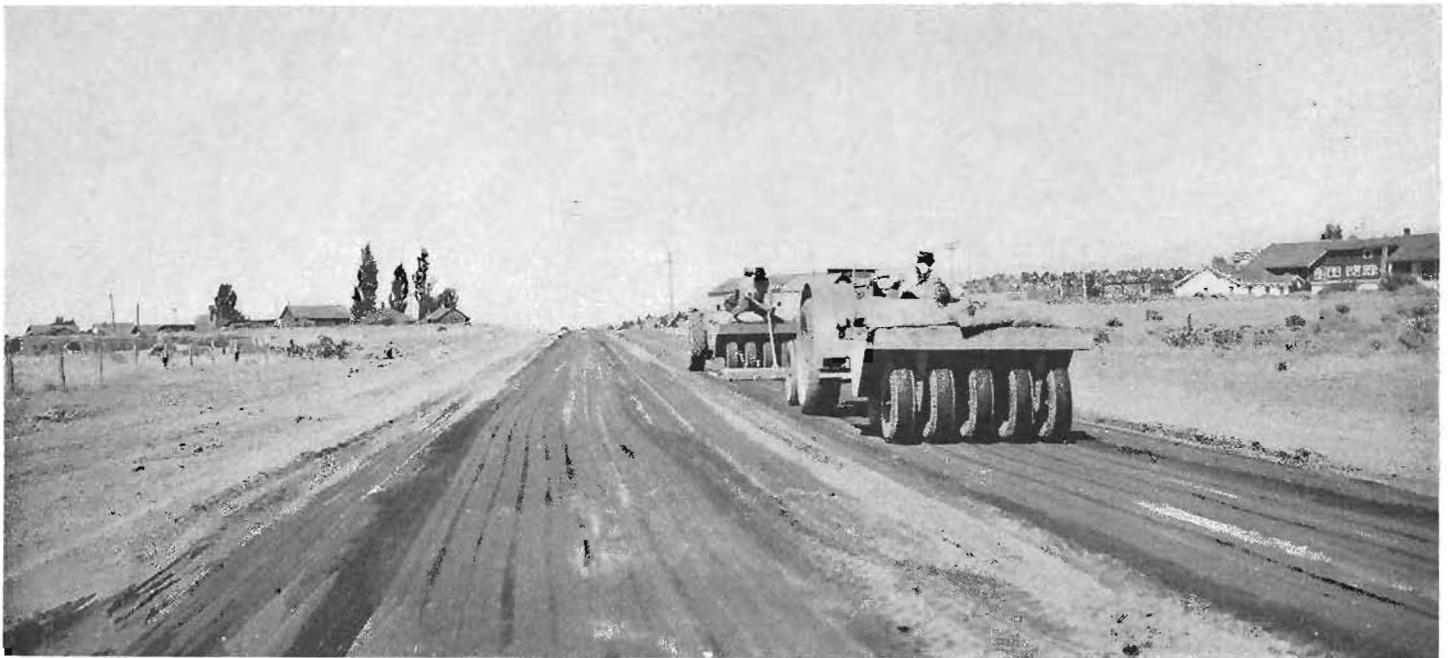
Tractors equipped with big rubber-tired wheels and weighted with bags of cement rolling soil-cement base construction.
