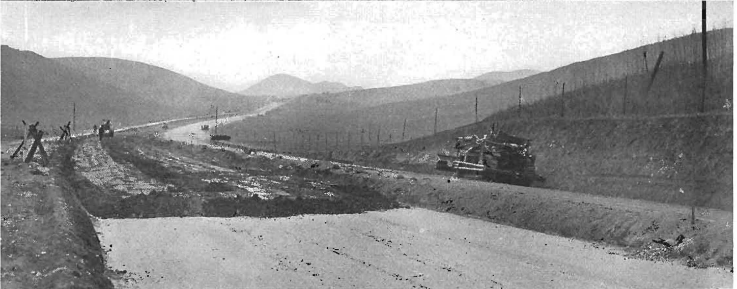
These pictures show three progressive operations in laying Portland cement concrete pavement. Upper—Membrane seal in place ready for imported borrow. Center—Motor grader spreading imported borrow over membrane seal. Lower—Imported borrow in place on membrane seal ready for grading and paving operations.
