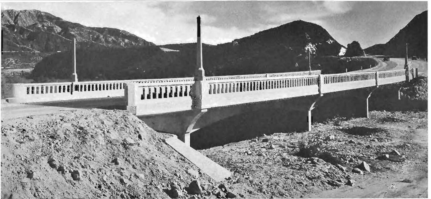
New concrete bridge over the south overflow channel of Big Tujunga Wash.
