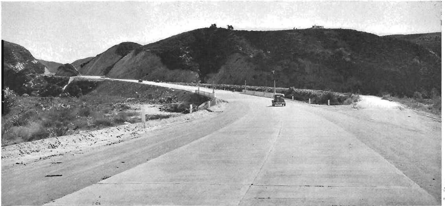
View easterly over new bridge across Big Tujunga Wash overflow channel. Old sharply curving alignment shown to right foreground and left background of new construction.
