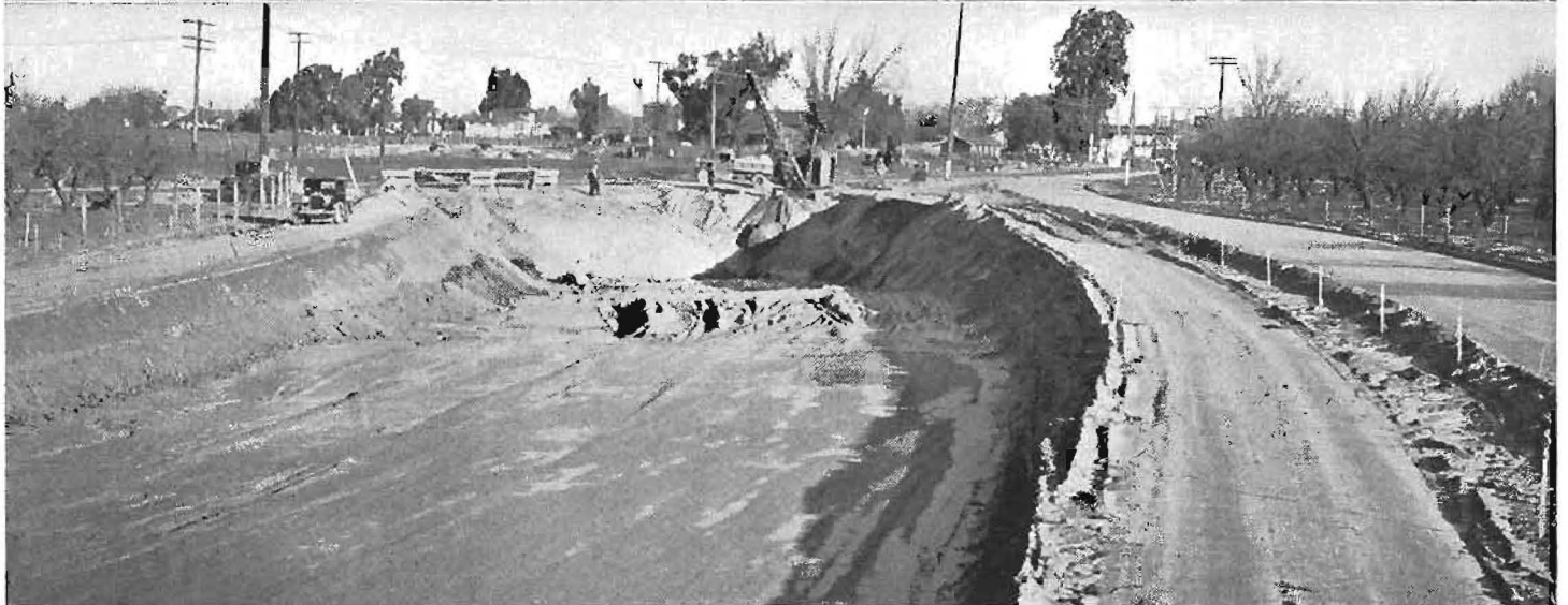
This "S"-turn grade crossing hazard in Livingston, Merced County, is being eliminated. Upper view shows railroad crossing looking southerly toward Livingston and center one shows traffic blockade caused by train. Lower—Excavation for Livingston underpass. Permanent detour on right.
