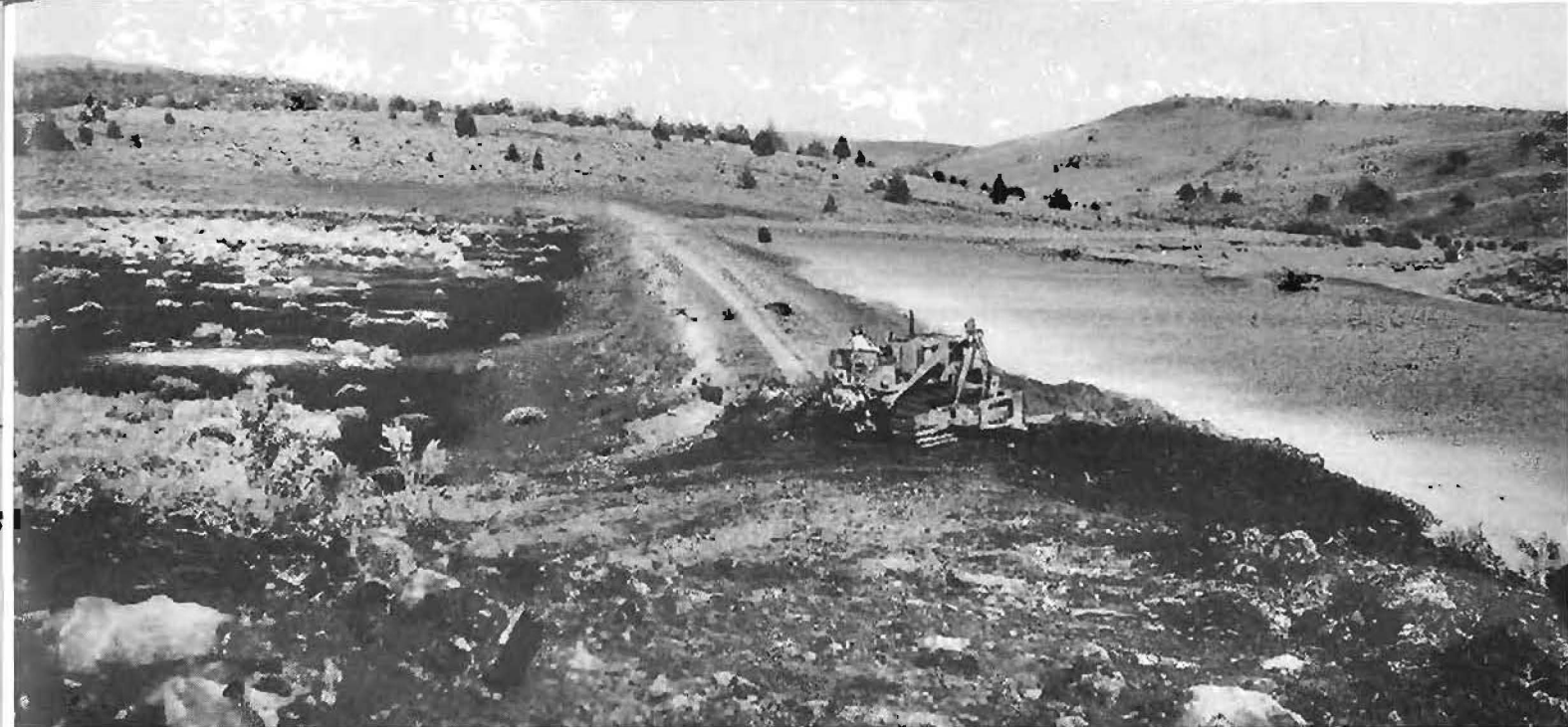
View of new Tule Lake Reservoir levee which was raised six feet under emergency construction to prevent its destruction and consequent wiping out of West Valley dam and flooding of Alturas.
