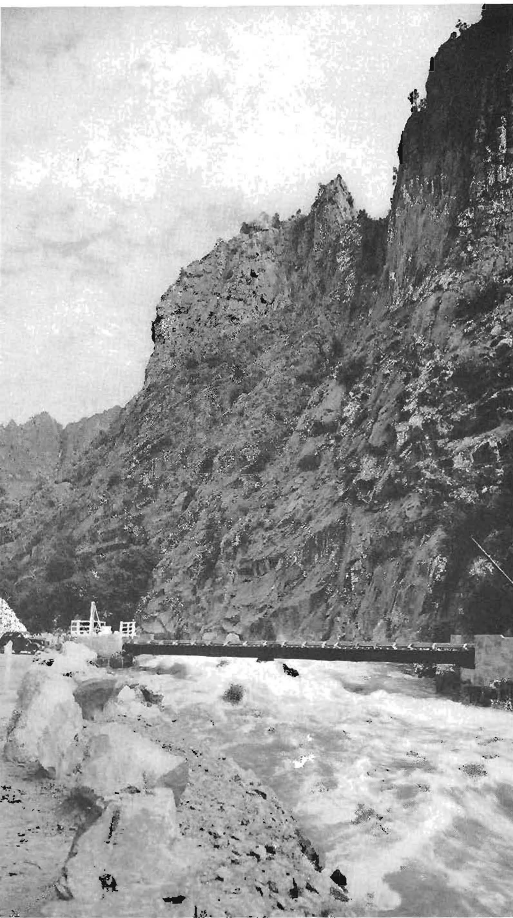
Kings River Bridge. Abutments and center pier complete. Superstructure half complete. Kings River, nearing flood stage, is roaring through canyon.
