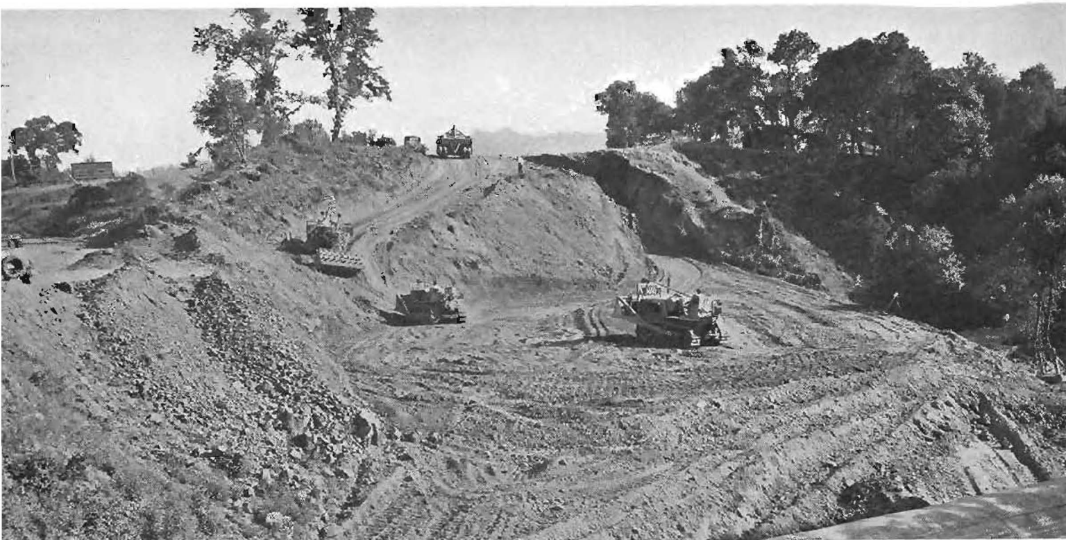
Heavy grading equipment in operation on Los Gatos-Inspiration Point link of new Santa Cruz Highway.
