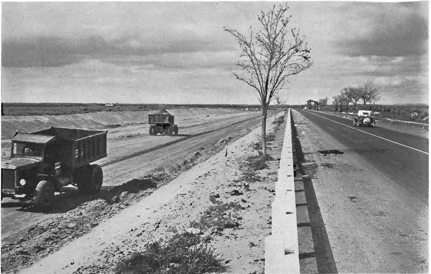
Contractor's trucks on new future southbound lane of Bakersfield-Grapevine Highway. Cars on present pavement which will be future northbound lane of four-lane divided highway now under construction.
