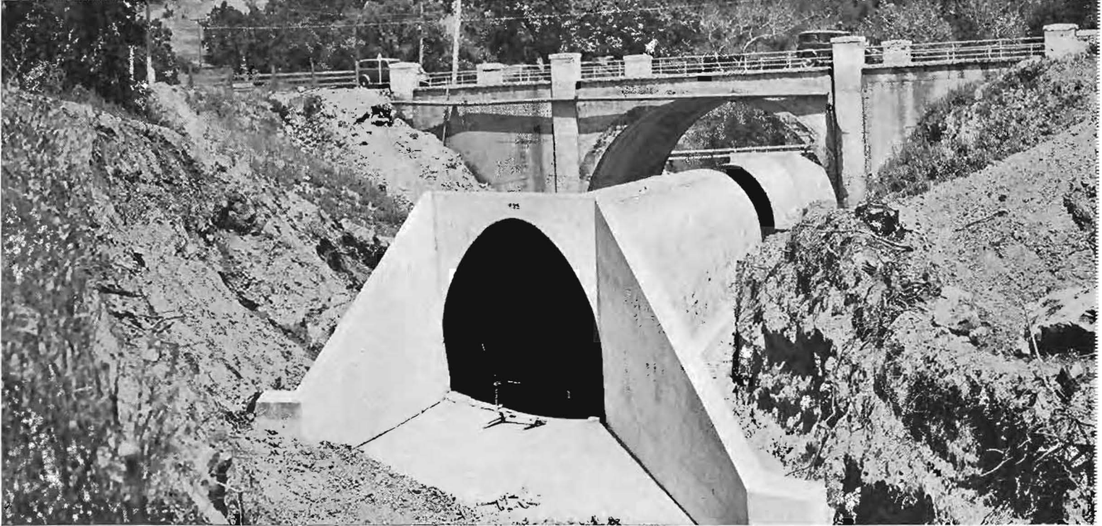
In upper picture is section of present winding Los Gatos-Santa Cruz Highway which is to be replaced by broad, straight road shown under construction in center. Lower—Portion of huge drainage system for new road.
