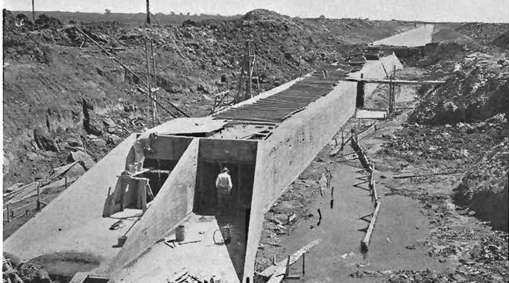
Construction view of Contra Costa Conduit showing syphon under county road and earth canal east of Oakley.
